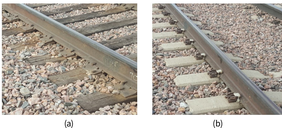
Figure 3-3 (a) Cut spikes in timber crossties; (b) elastic fasteners on concrete crossties
