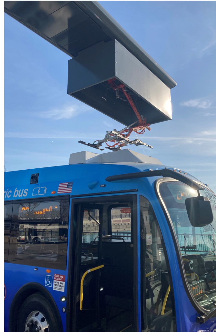
Figure 4 - Photo of pantograph charger at Navy Pier
