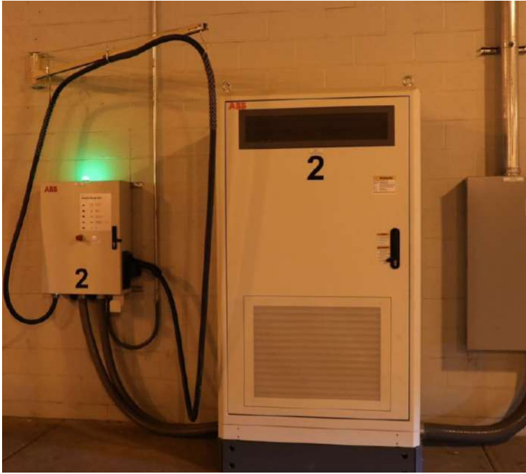
Figure 6.3: ABB Level 2 charger and dispenser at CTtransit New Haven
