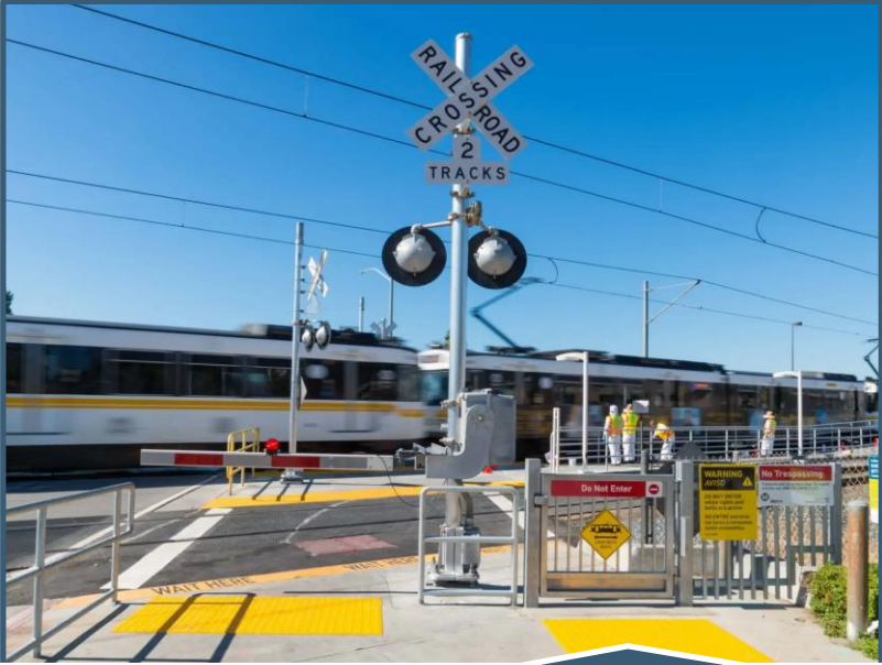
Rail Crossing Gates
