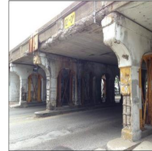
Crumbling viaduct at Hollywood Ave.
