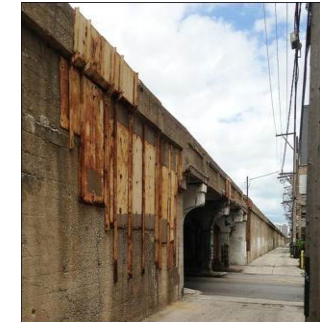
Crumbling retaining wall near Bryn Mawr
