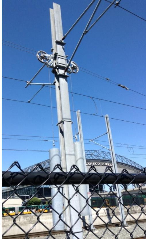
Figure 4. Auto-tension Weights for Overhead Catenary Systems. The self-adjusting cylindrical weights are hanging on either side of the support pole. Photo source: Sound Transit.
