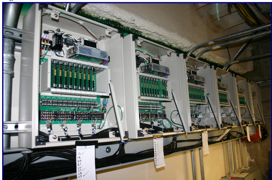
Figure 6: RIAS Controller Unit
