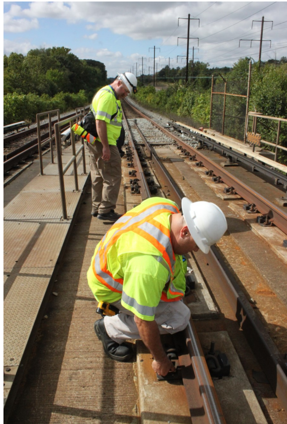
FTA investigators Phil Herbert (left) and Troy Lloyd (right) examine a section of WMATA Metrorail track.
