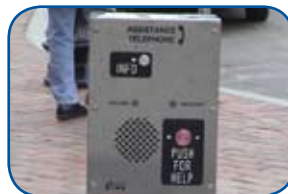
Passenger Security Phone at bus stop
