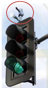
Figure 4-23: Opticom Strobe Detector
