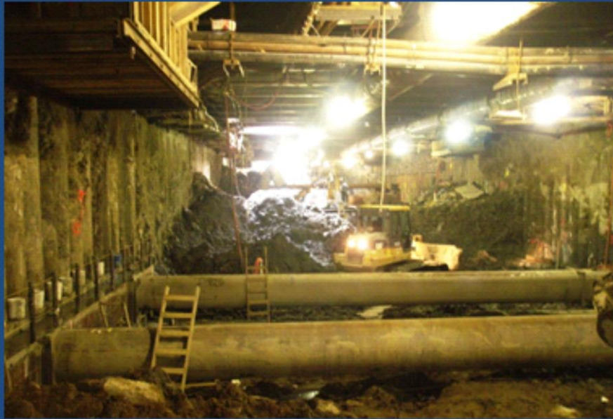
92 nd – 93 rd St: Installation of wale W-5 and associated struts (looking South)
