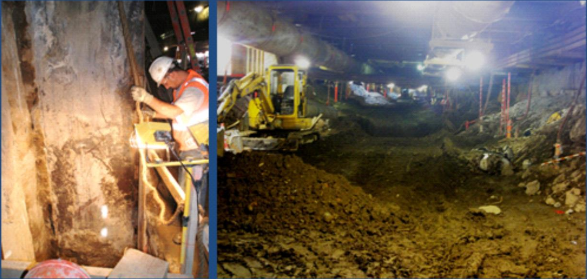
93 rd - 94 th St: Exposing joint at Secant Pile/Slurry wall interface (left); Excavation progress looking south (right)
