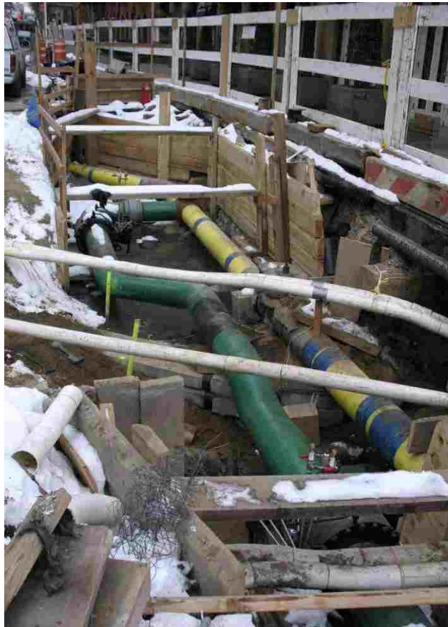
Installation of 12" HP Gas Main -- NW Corner of 96 th St. and 2 nd Ave.
