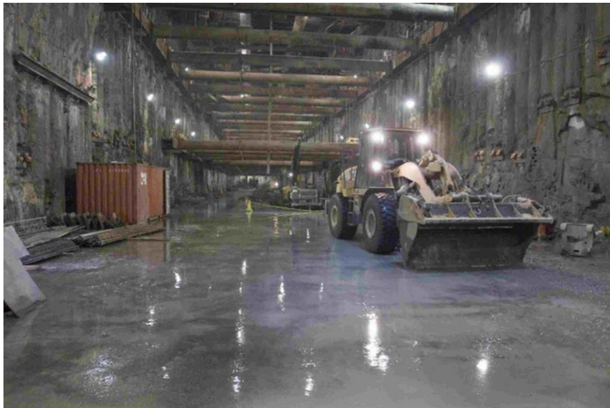
This photo shows the tunnel boring machine launch box underneath Second Avenue between 91st and 95th Streets.
