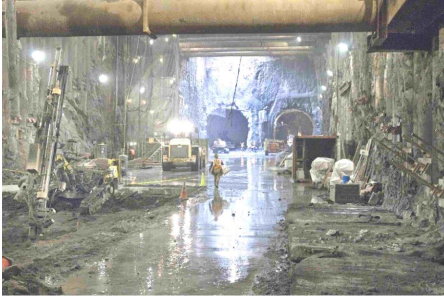
This photo shows the tunnel boring machine launch box underneath Second Avenue between 91st and 95th Streets. At rear of photo are the tunnel boring machine starter tunnels.
