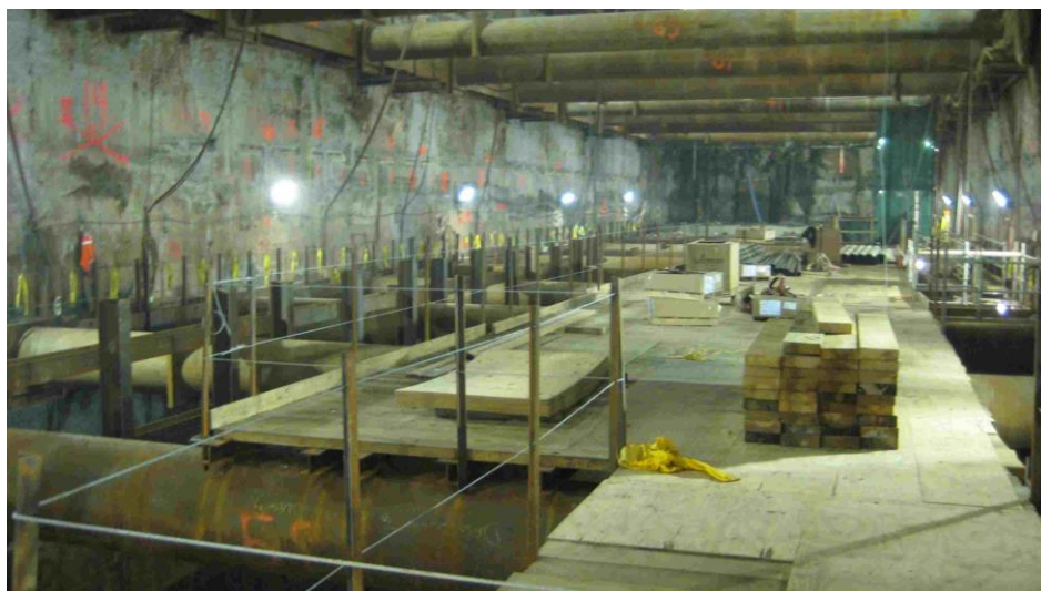
94th-95th St: Continued construction of muck bin observation deck at Tier 3 bracing level
