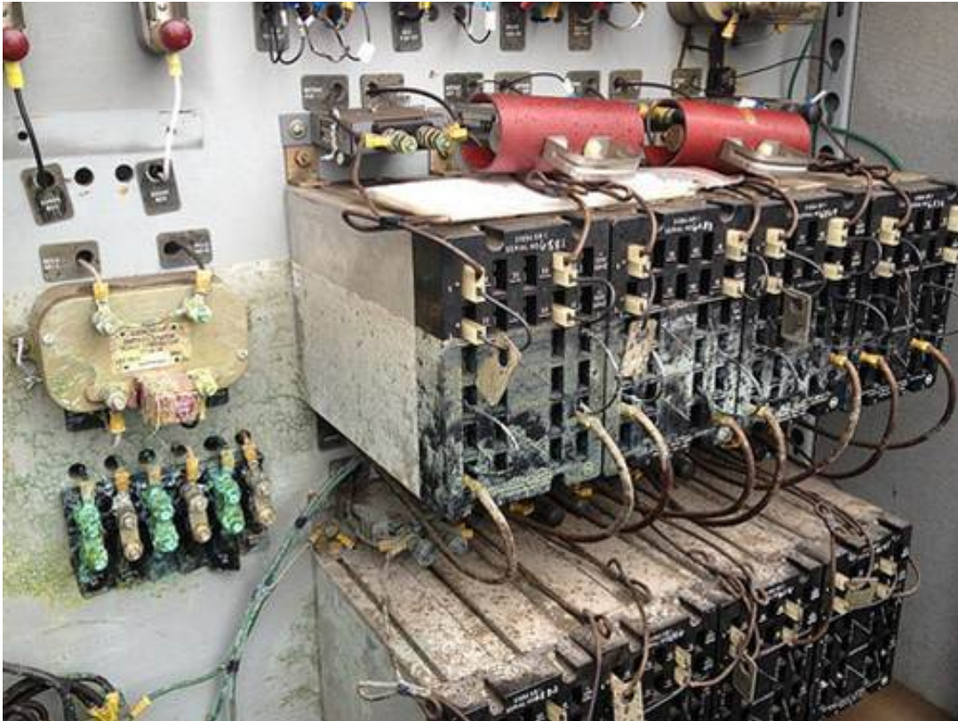
Corroded MTA equipment from Hurricane Sandy, New York, NY - 2013
