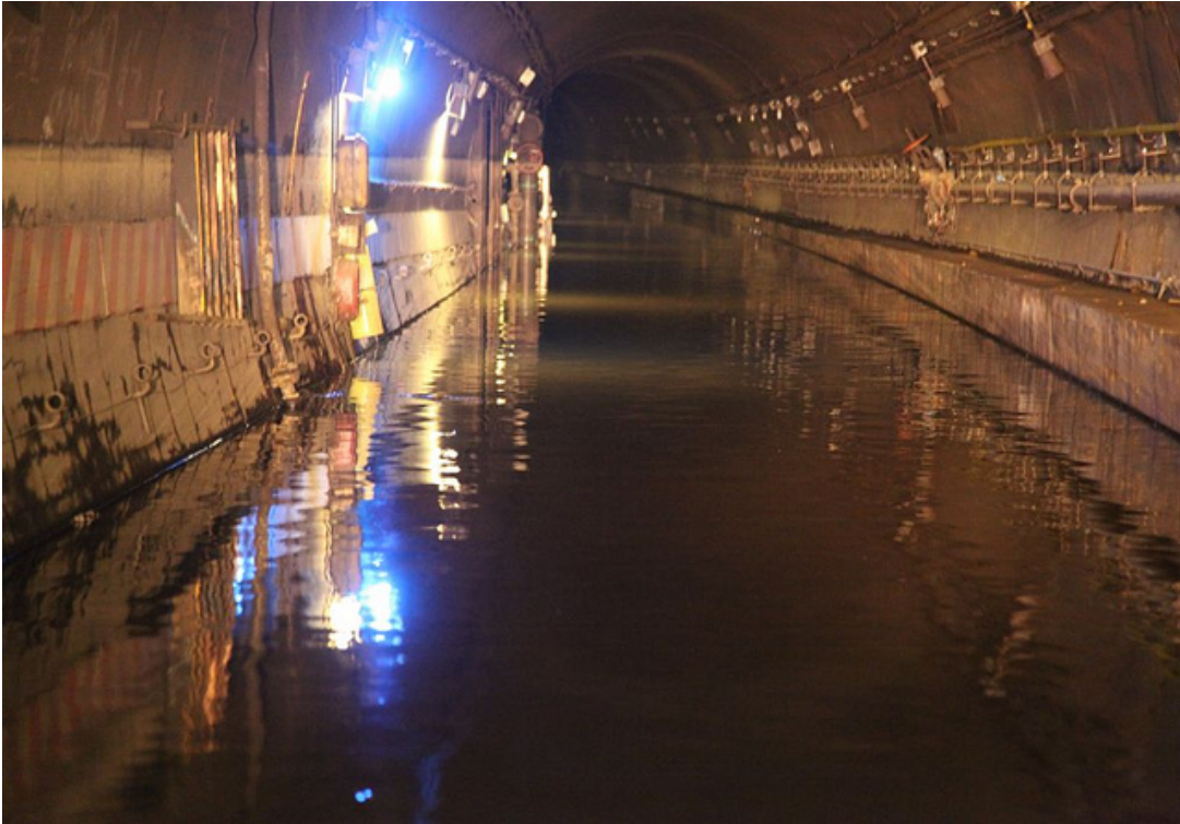
Hurricane Sandy flooding, New York, NY - 2013
