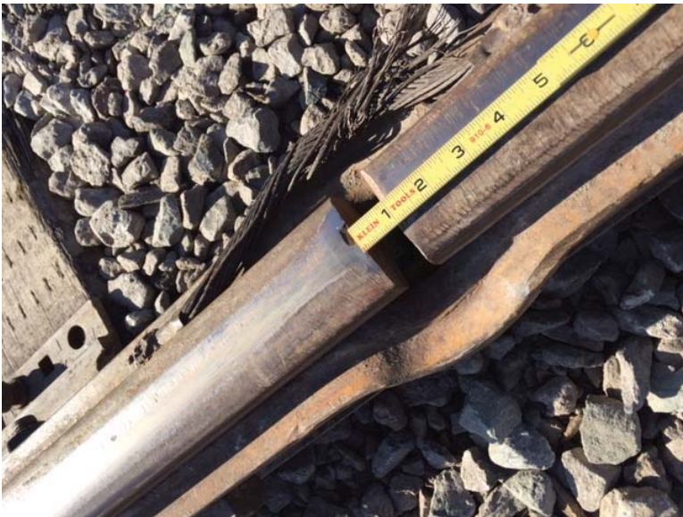
Figure 2: One-inch gap between rail running surfaces at B2 294+80, right rail.
