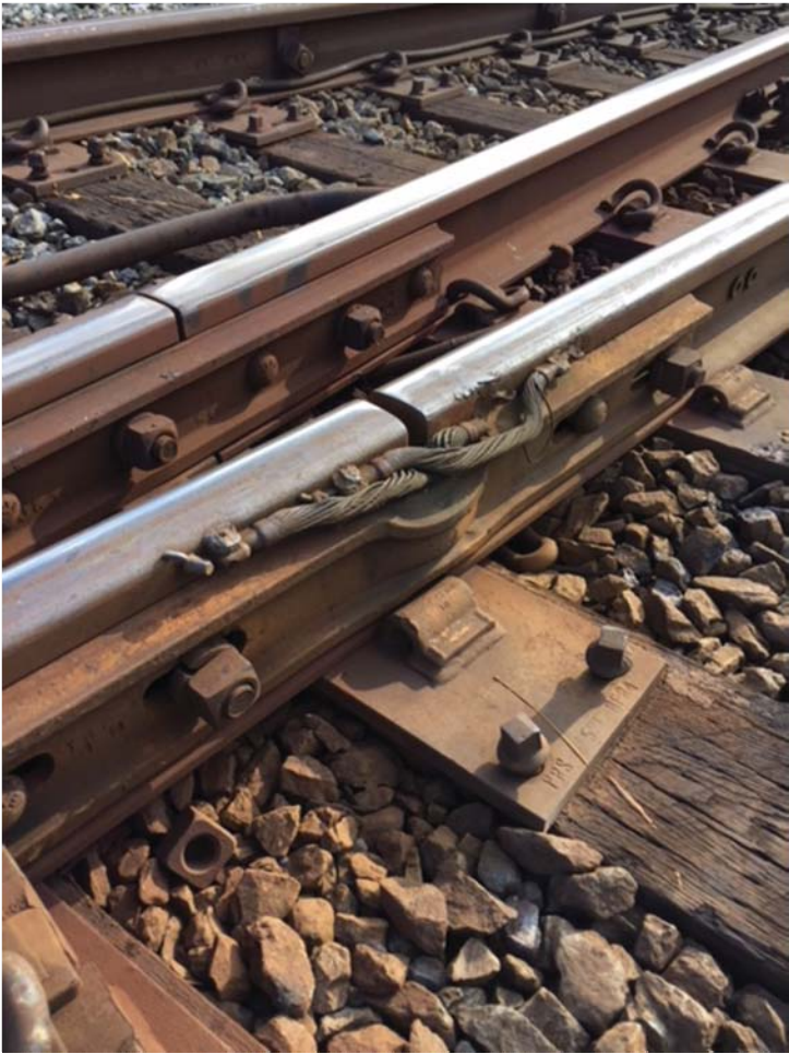
Figure 1: Incorrect joint bar and missing Pandrol clips at B2 258+00. 3B switch.
