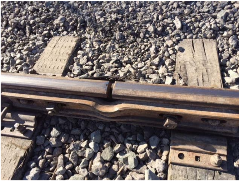
Figure 1: Improper joint bar at B2 294+80, right rail.
