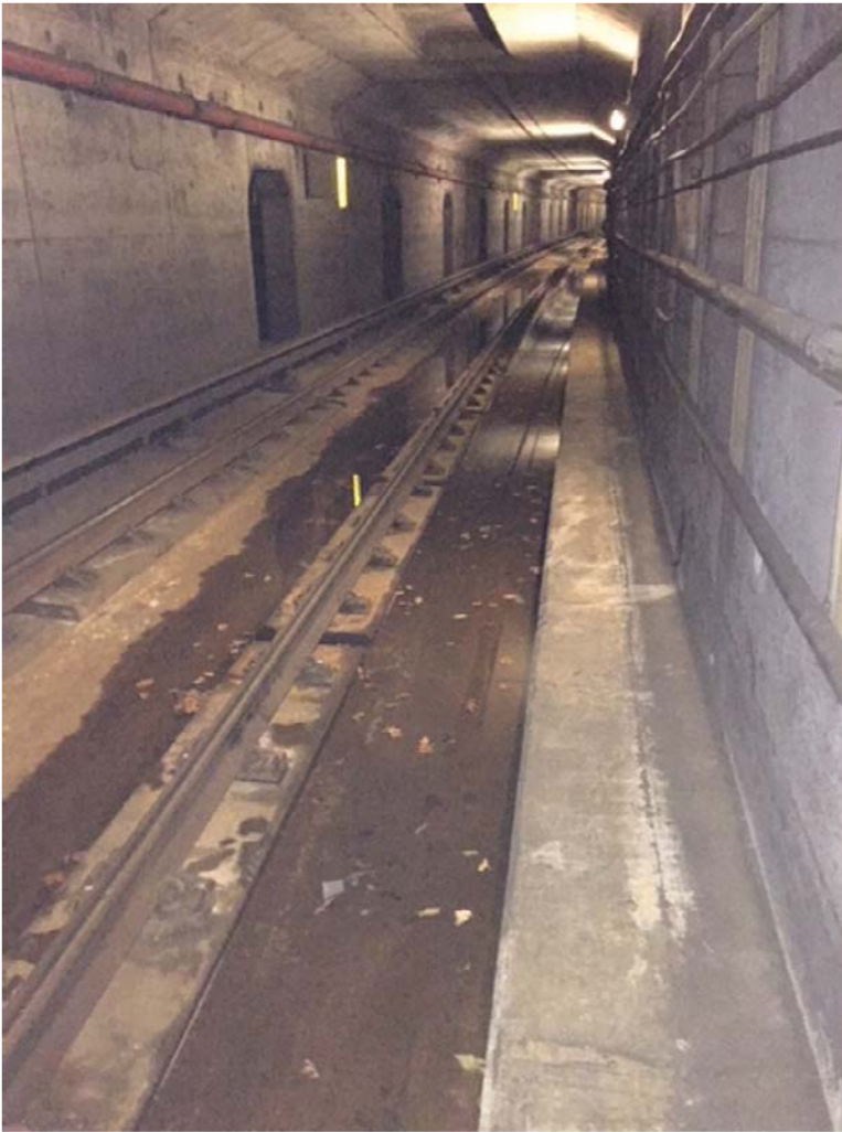
Figure 1: Blocked drains not draining as designed and allowing pooling water at F1 338+00.
