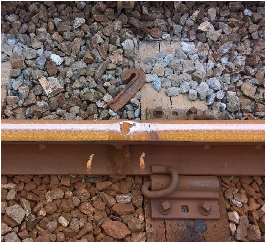
Figure 1: Chipped rail at CM B2 086+00.
