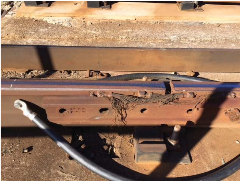
Figure 1: Missing bolts on the left rail joint at D2 468+20
