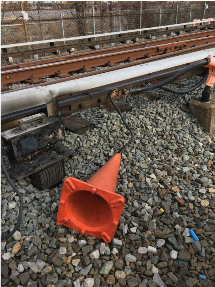
Figure 1: Unsecured wire at J2 567+00.
