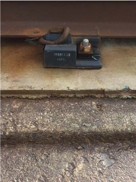
Figure 3: Fastener not seated to the grout pad on the New Carrollton aerial structure.
