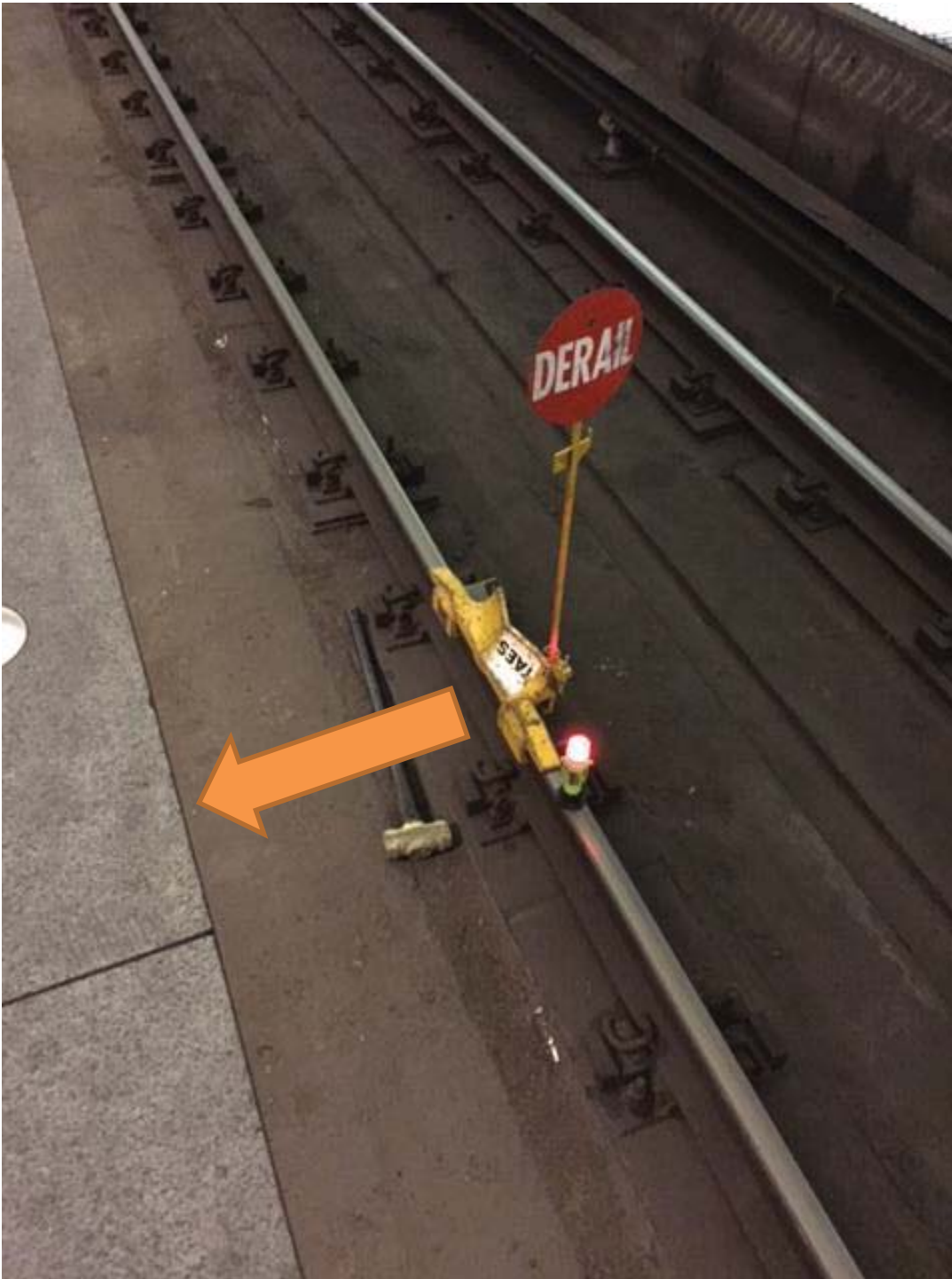
Figure 1: Derailed located at A2 444+30 installed to derail a train in the direction indicated by the arrow.
