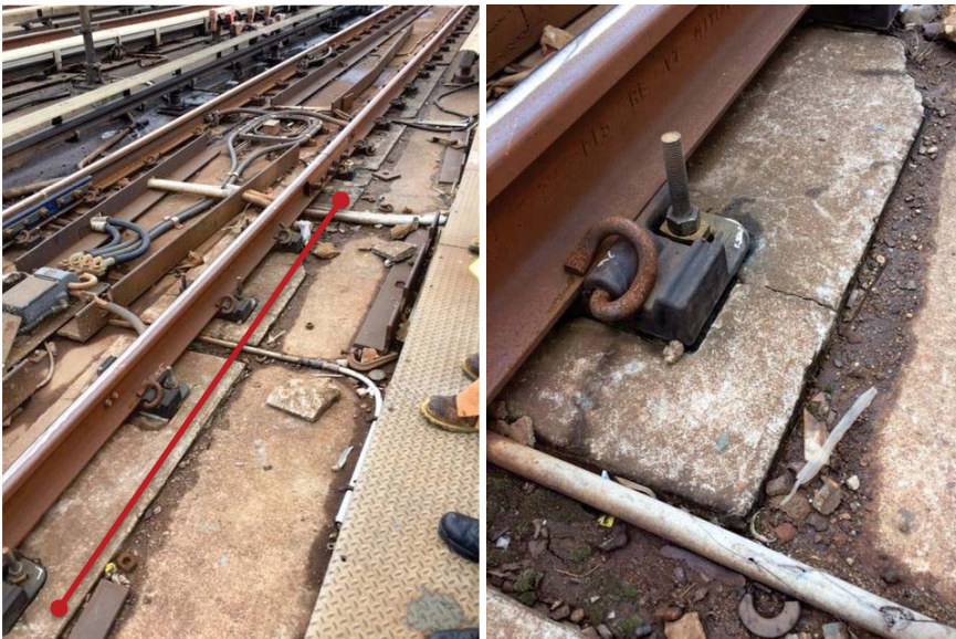
Figures 4 and 5: Five consecutive non-holding fasteners with 3/8-inch dynamic movement at D2 285+00 at the D98-52 signal.
