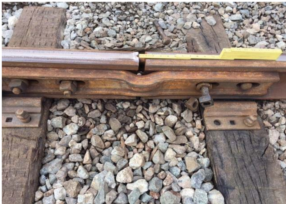
Figure 2: Improper joint bar and loose bolt at D2 294+80.
