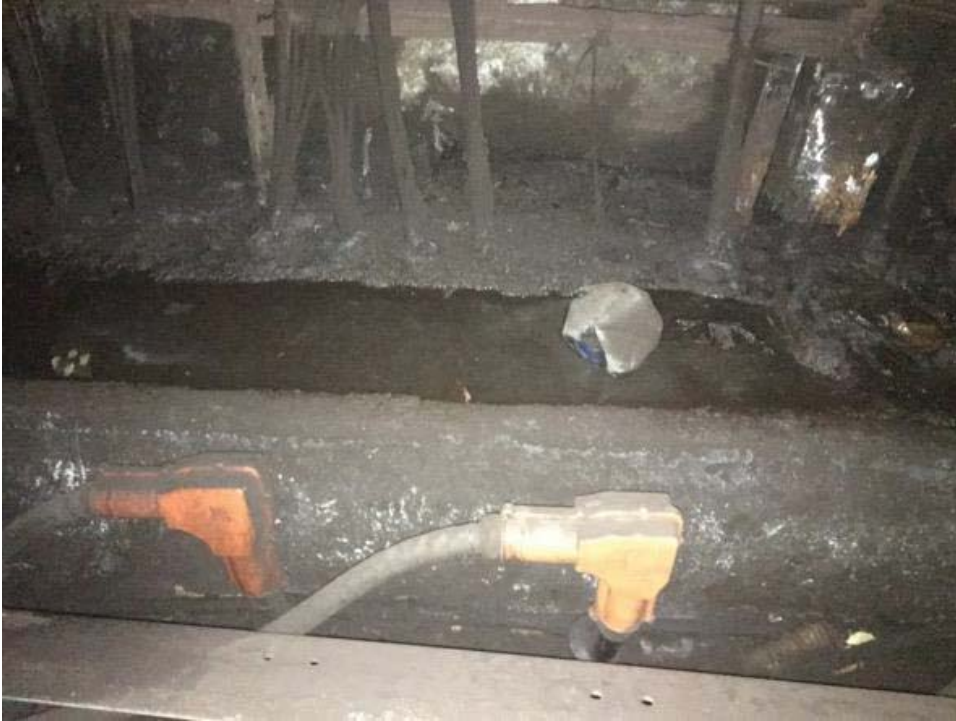
Figure 1: Standing water above orange boot cable connector assemblies from A1 304+00 to A1 309+00.
