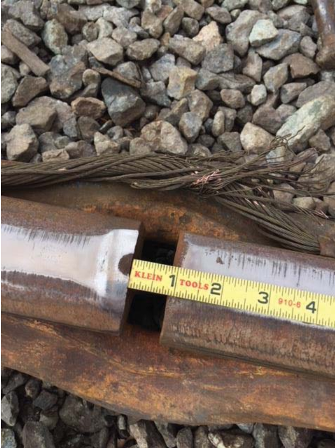
Figure 1: A 7/8-inch gap in running surface at D2 294+80.
