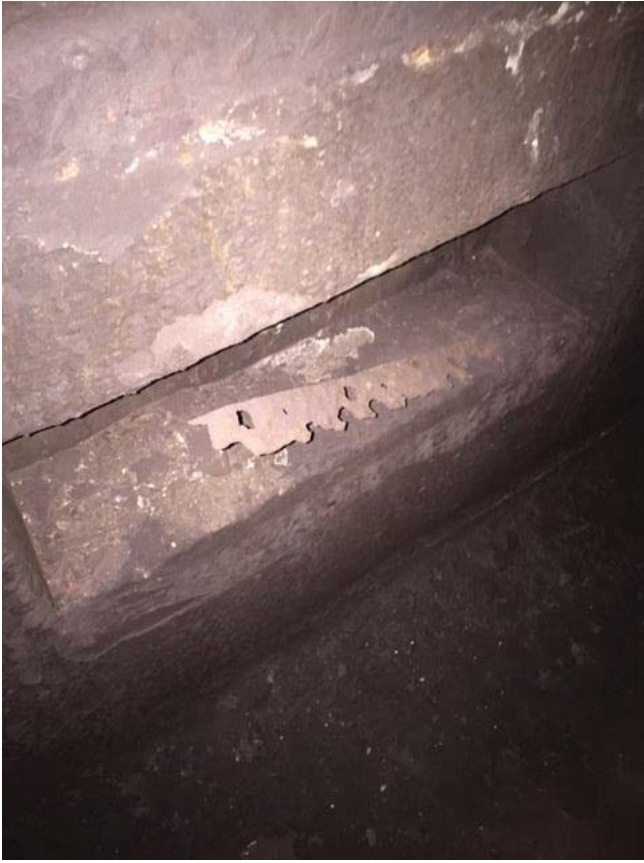
Figure 2: At A2 372+00, the diamond plating has rusted and was detaching
