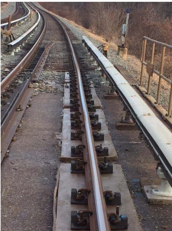
Figure 2: Spike misalignment at D1 477+80, right rail.
