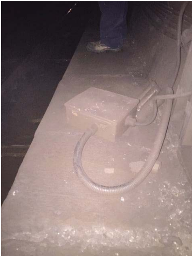
Figure 1: At A2 308+90, the electrical junction box dislodged from the wall and lying on the catwalk.
