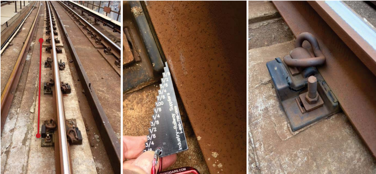
Figures 1, 2 and 3: Five consecutive non-holding fasteners with 5/8-inch dynamic movement and 56 3/4 dynamic gauge at D2 260+30.
