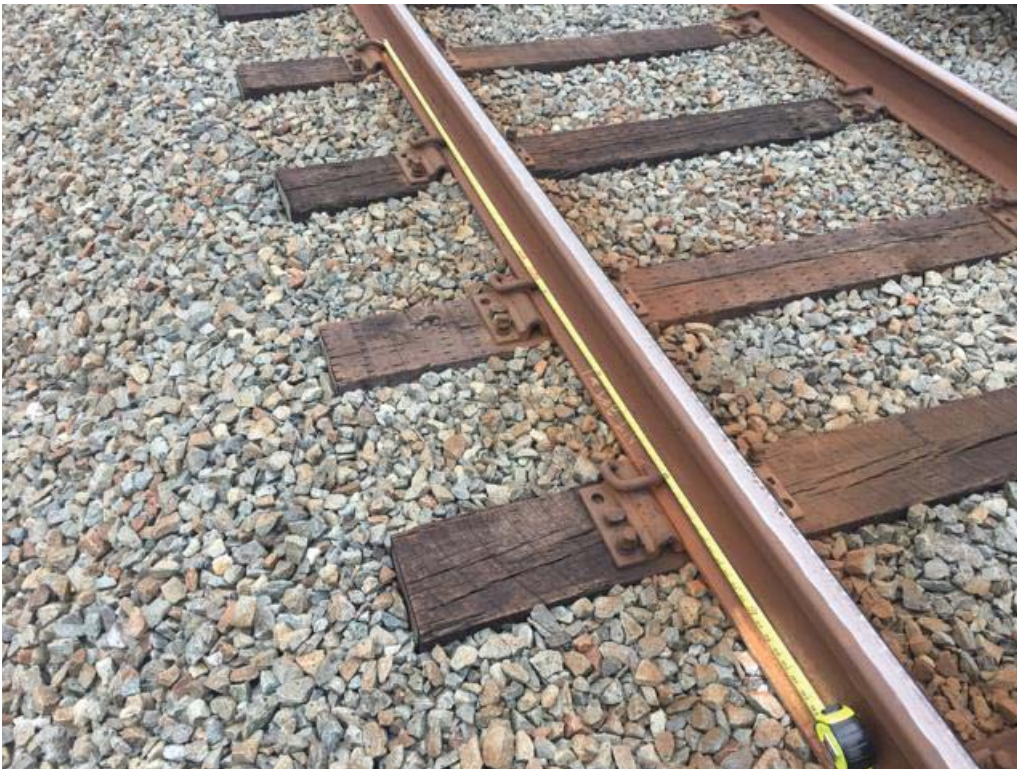
Figure 2: Non-Testable Rail, right rail eight feet in length at J1 856+50.
