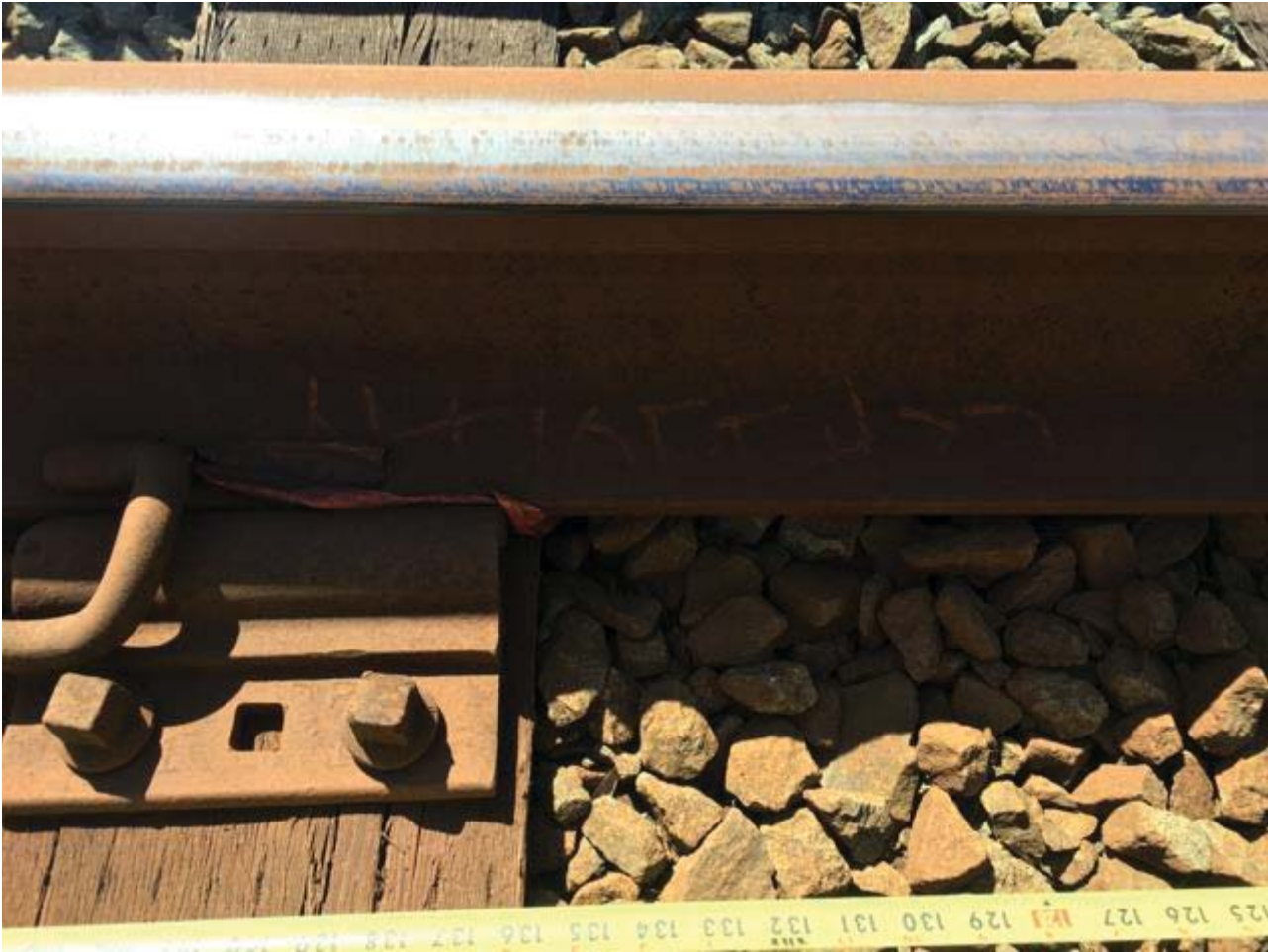
Figure 2: Non-Testable Rail, left rail and high rail of curve at 687+80.
