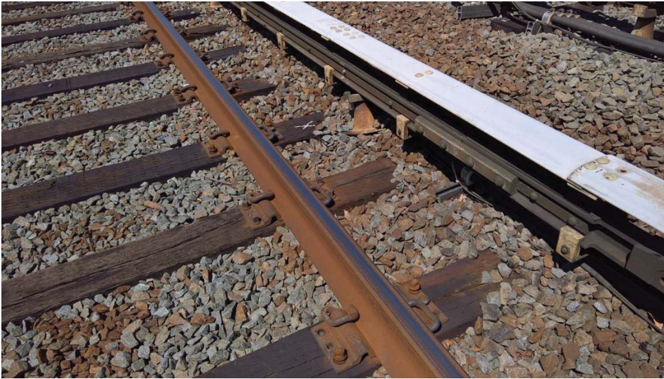
Figure 2: Third rail insulators at CM F2 427+50 to CM F2 428+50.
