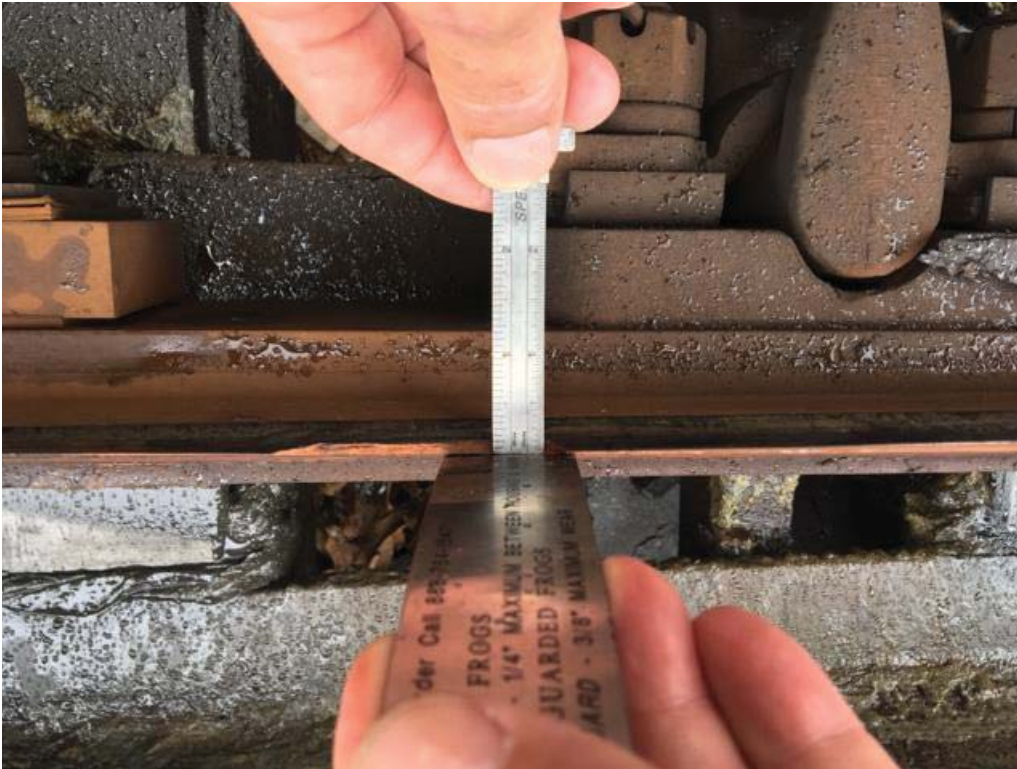
Figure 1: Chipped Point (Width 1/8") Right hand point, turnout side 1A switch at J1 874+00.
