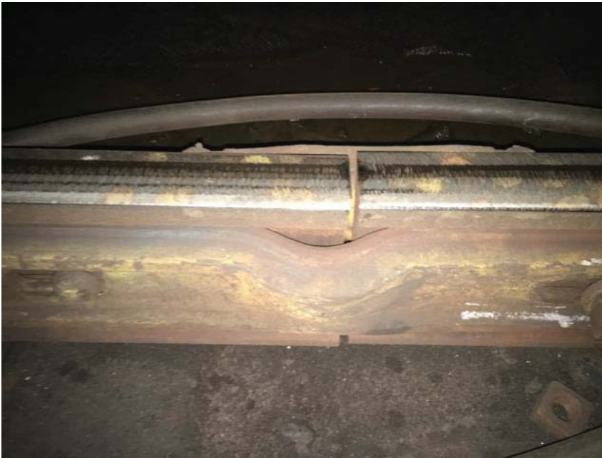
Figure 1: Improper joint bar was installed at the rail joint, right rail at 105+00. These bars are not designed to provide the same structural contact fitting into the web with contact along all sides of the base and underside of the ball. These are also designed with slotted bolt holes allowing excessive movement which affect RNT and opens the joint producing significant impact. They don't restrain the rail since the joint can open 2 inches as the bolt slides through the slots. They are designed to give additional protection to a field weld so if it breaks the rails stay lined up.
