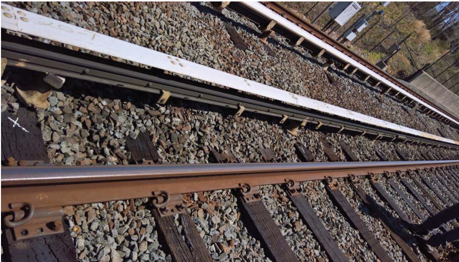
Figure 1: Third rail insulators at CM F2 427+50 to CM F2 428+50.
