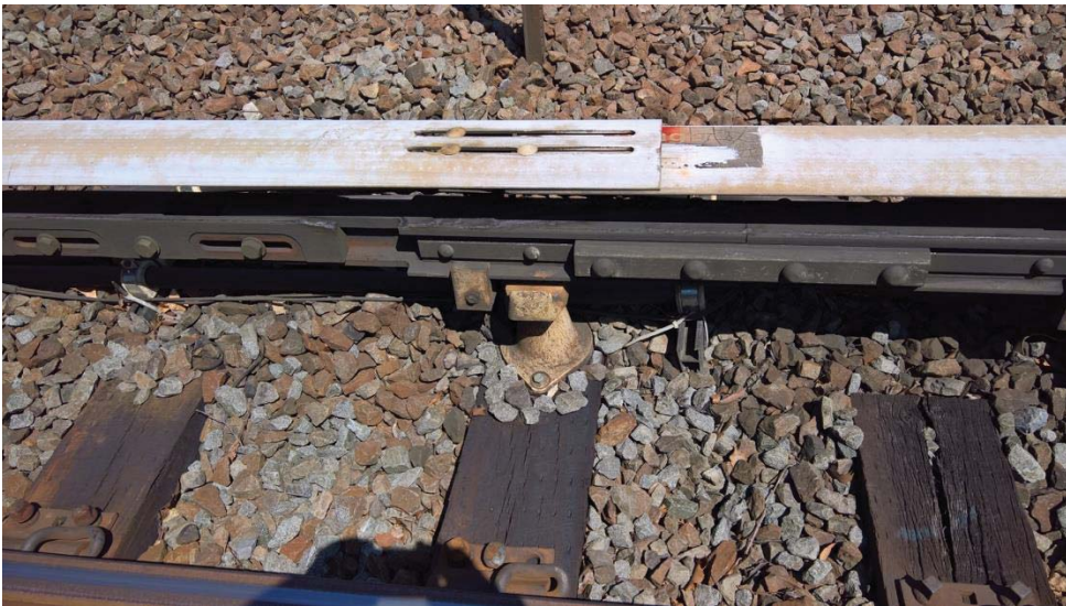
Figure 3: Third rail insulators at CM F2 427+50 to CM F2 428+50.
