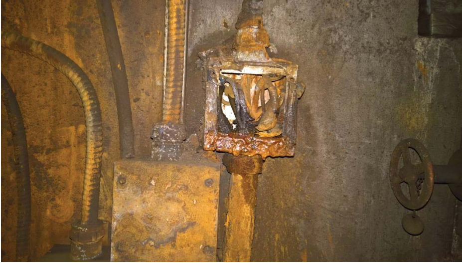
Figure 1: CM 249+30 tunnel leak through electric box.
