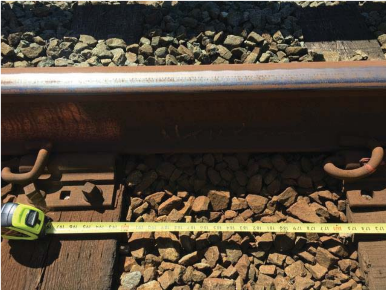
Figure 1: Non-Testable Rail, sixteen feet in length, left rail and high rail of curve at 689+50.
