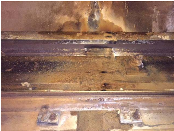
Figure 1: Sidewall tunnel leak at CM C1 635+00.
