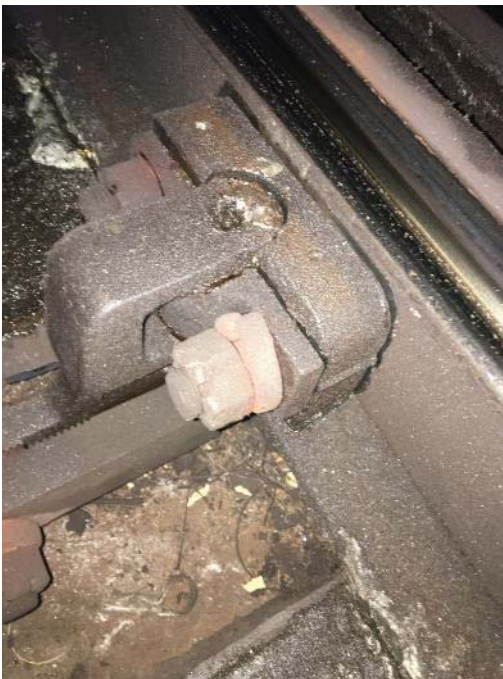
Figure 2: Loose bolts at C2 571+80 on #4 switch.
