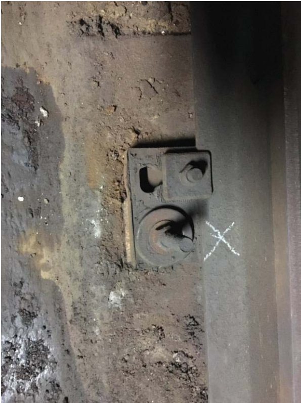
Figure 1: Defective fastener at D1 117+90, ID # 2123 has ¼" movement underload.
