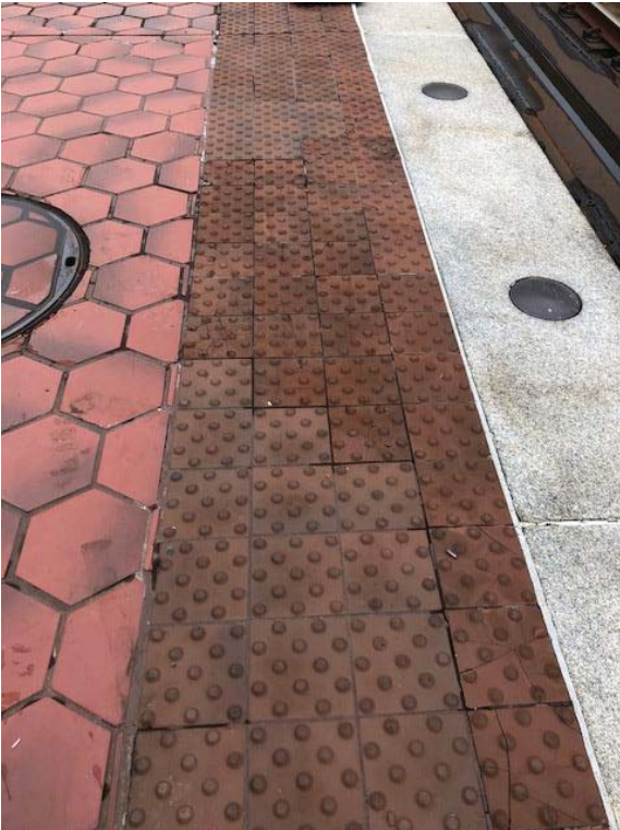
Figure 2: Dislodged pavers at Van Dorn Street platform track two side.
