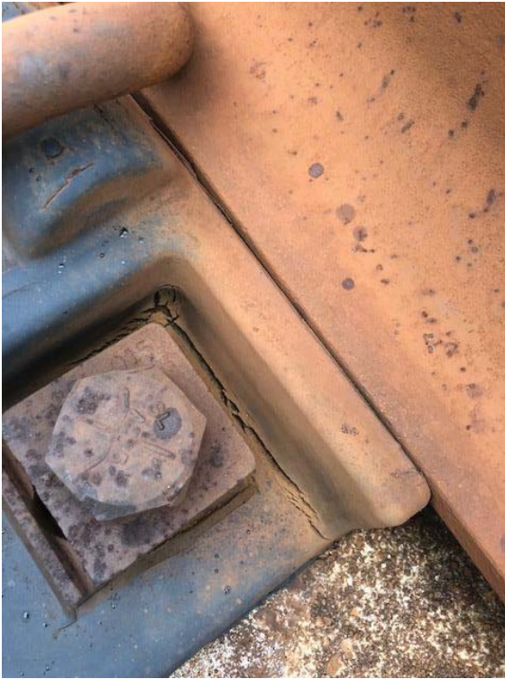
Figure 3: Failing elastic fasteners on track two within the three aerial structures.
