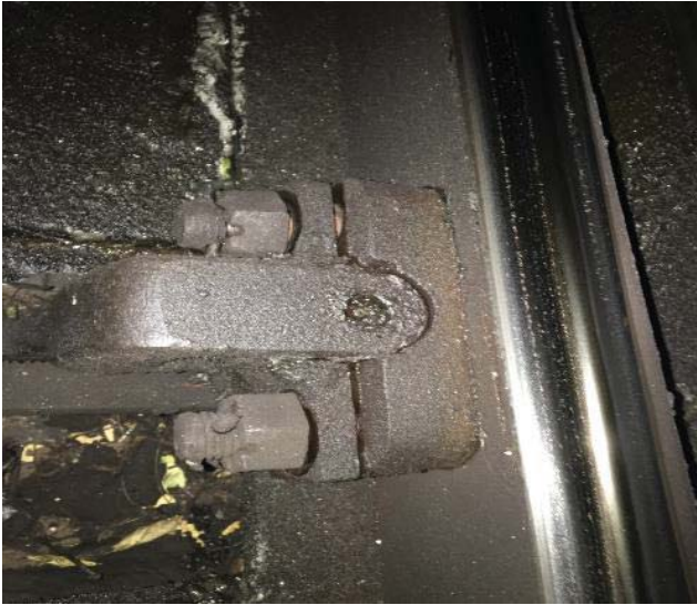
Figure 1: Loose bolts at C2 751 + 80 on the # 3 rod.
