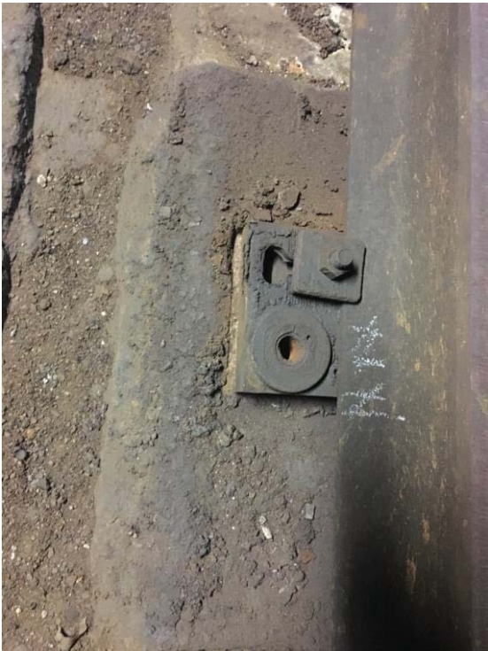
Figure 2: Defective fastener at D1 117+90, ID # 2123 has ¼" movement underload.
