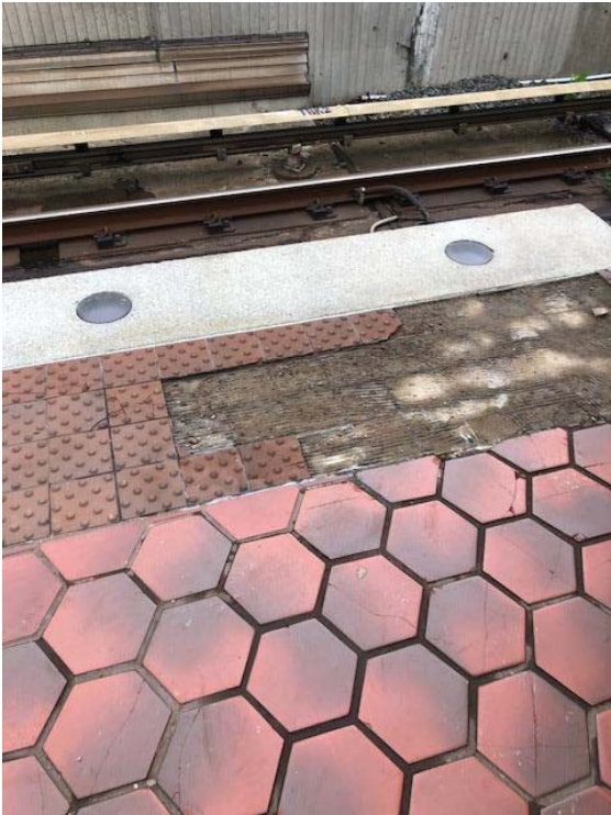
Figure 1: Dislodged pavers at Van Dorn Street platform track two side.
