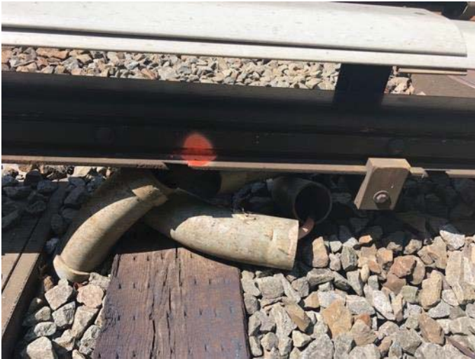
Figure 1: Cables underneath third rail at F1 408+50.
