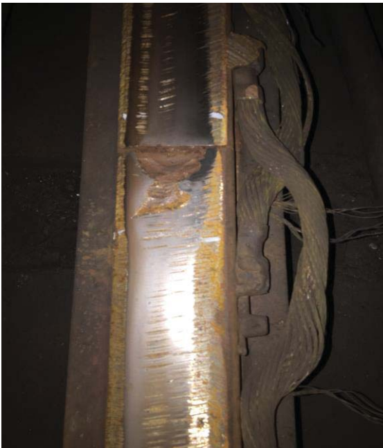
Figure 2: 3/16 inch mismatch at joint at D1 085+80.
