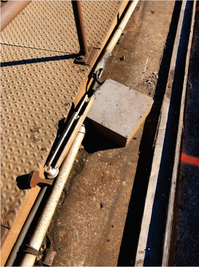
Figure 3: Dislodged electrical junction box at D1 261+40.
