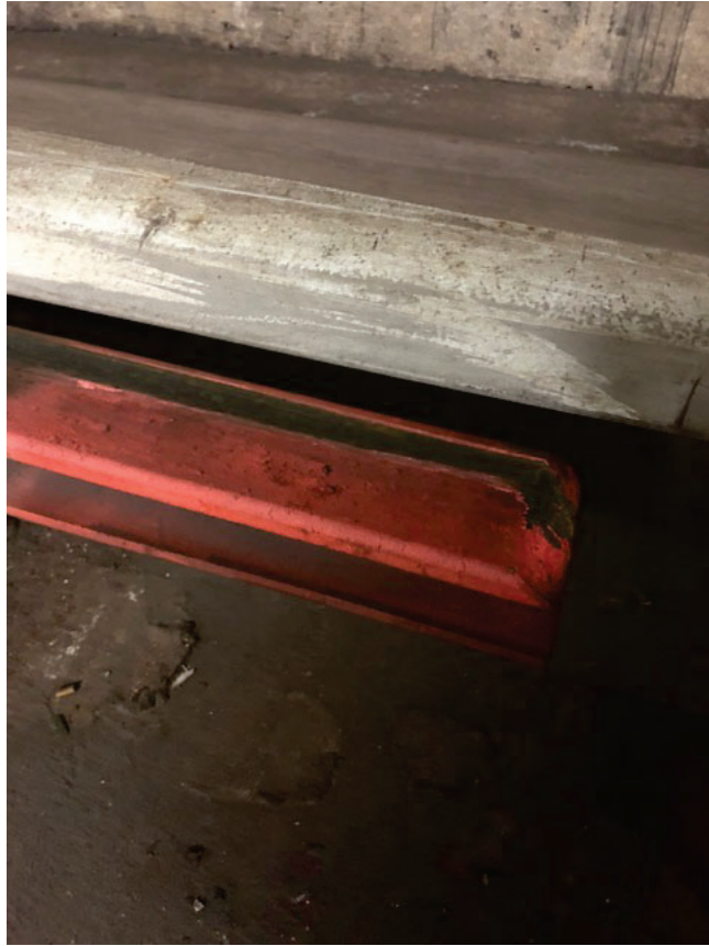
Figure 4: Collector shoe strike marks at D1 212+30 end approach.
