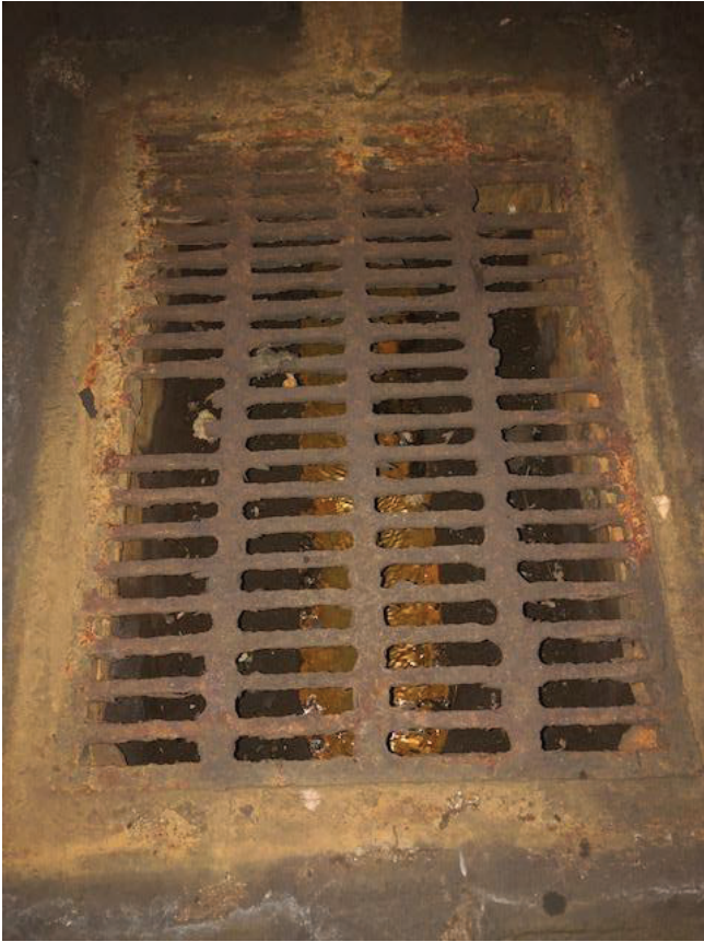
Figure 3: Deteriorated and corroded center drain at F2 033+25.
