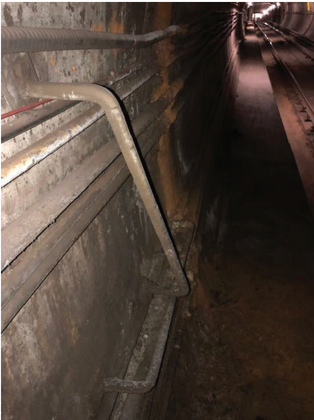
Figure 1: Dislodged hand railing at F2 038+00.
