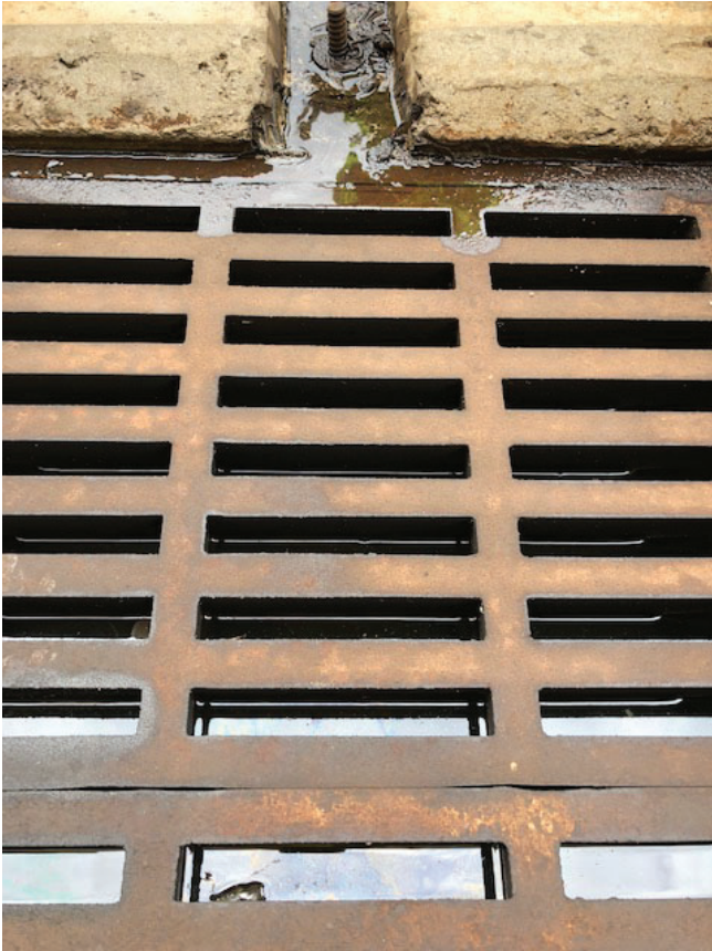
Figure 1: Blocked center drain at N2 698+00.
