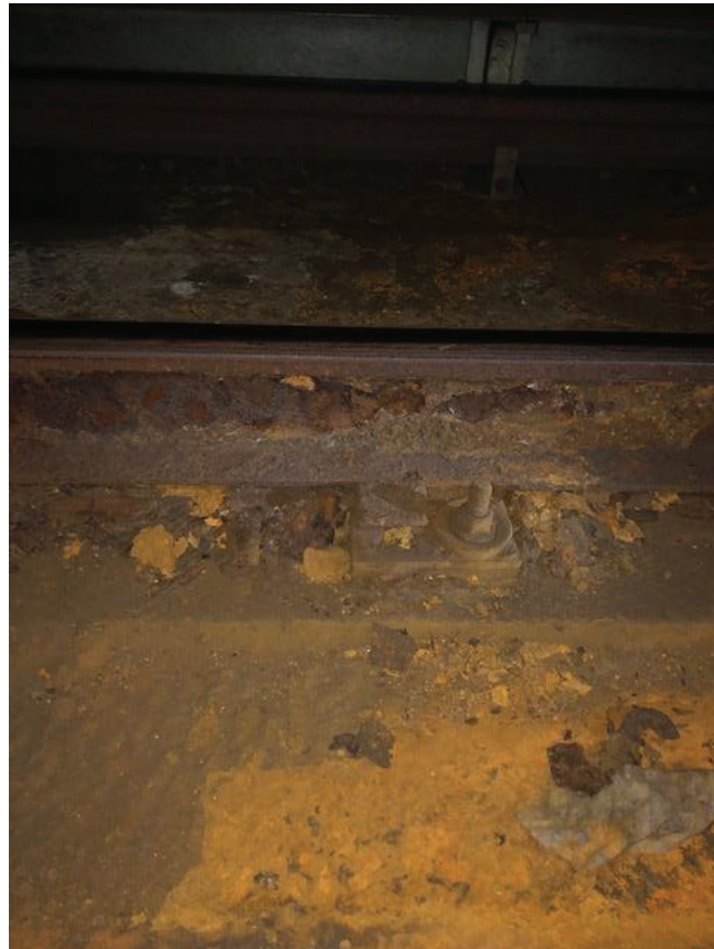
Figure 2: Web corrosion on the right rail at F2 035+35.
