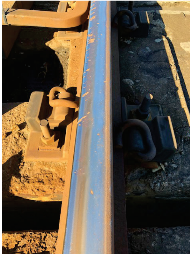
Figure 2: Rail spalling at D1 272+00.
