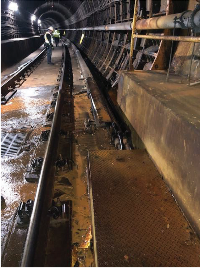
Figure 1: Tunnel leak at L2 070+60.
