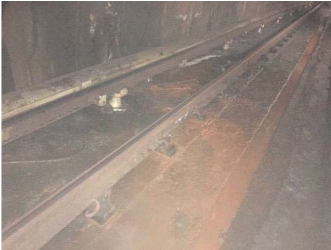
FIGURE 7 – A1 056+00 - DAMAGED CABLE FROM RUBBING AGAINST 3 RD RAIL COVER BOARD
