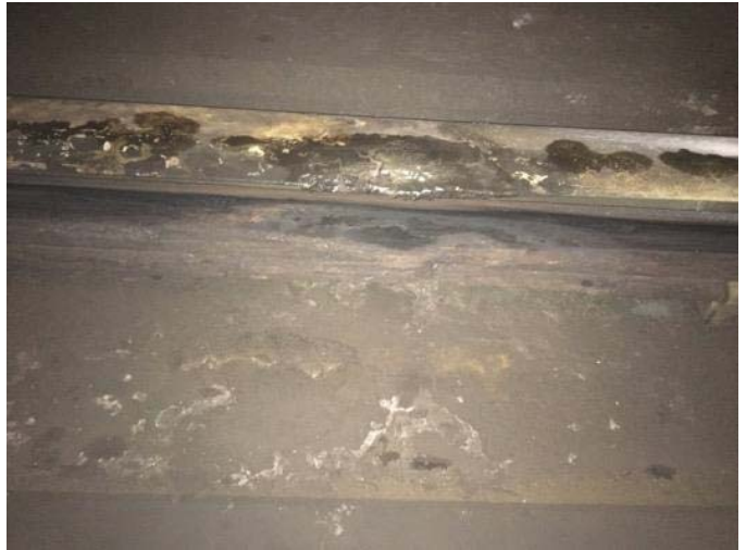
FIGURE 8 – A1 056+00 - DAMAGED ORANGE BOOT FROM RUBBING AGAINST 3 RD RAIL COVER BOARD
