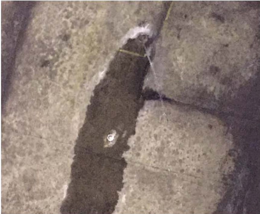
Figure 3: Water draining from another bored hole.
