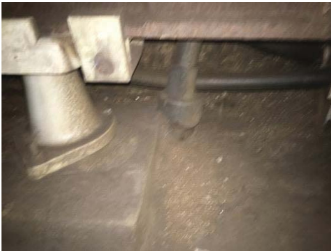
FIGURE 3 – A1 046+00 - CABLE JACKET NICKED
