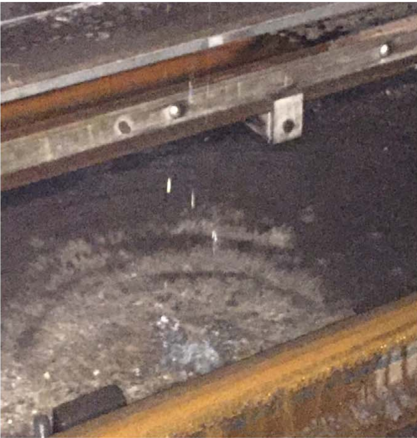
Figure 4: Pooling water from a bored hole accumulating on tunnel floor at the base of the rail.
