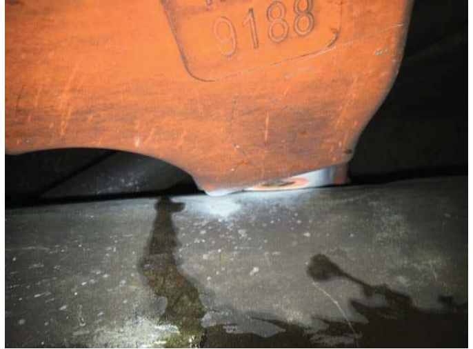
FIGURE 6 – A1 055+50 - PHYSICAL 3 RD RAIL RUSTED OUT AND WATER LEAKING FROM CEILING ONTO 3 RD RAIL COVER BOARD
