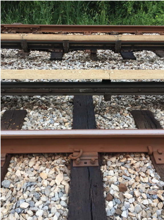
Figure 3: Newly installed 10-foot cross-tie without a third rail insulator support attached at E1 411+60.
