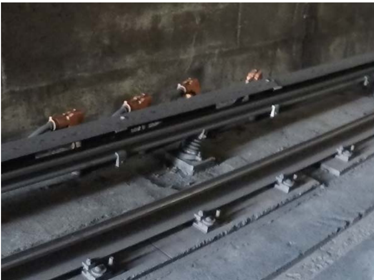
Figure 3: Broken insulator at G1 295+30.
