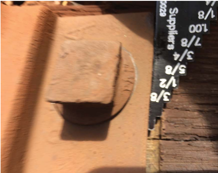
Figure 1: 1/4-inch field side dynamic plate movement at F2 401+00.
