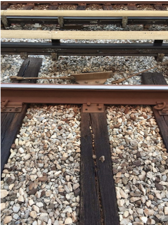
Figure 4: Disconnected third rail cable support at E1 406+60.
