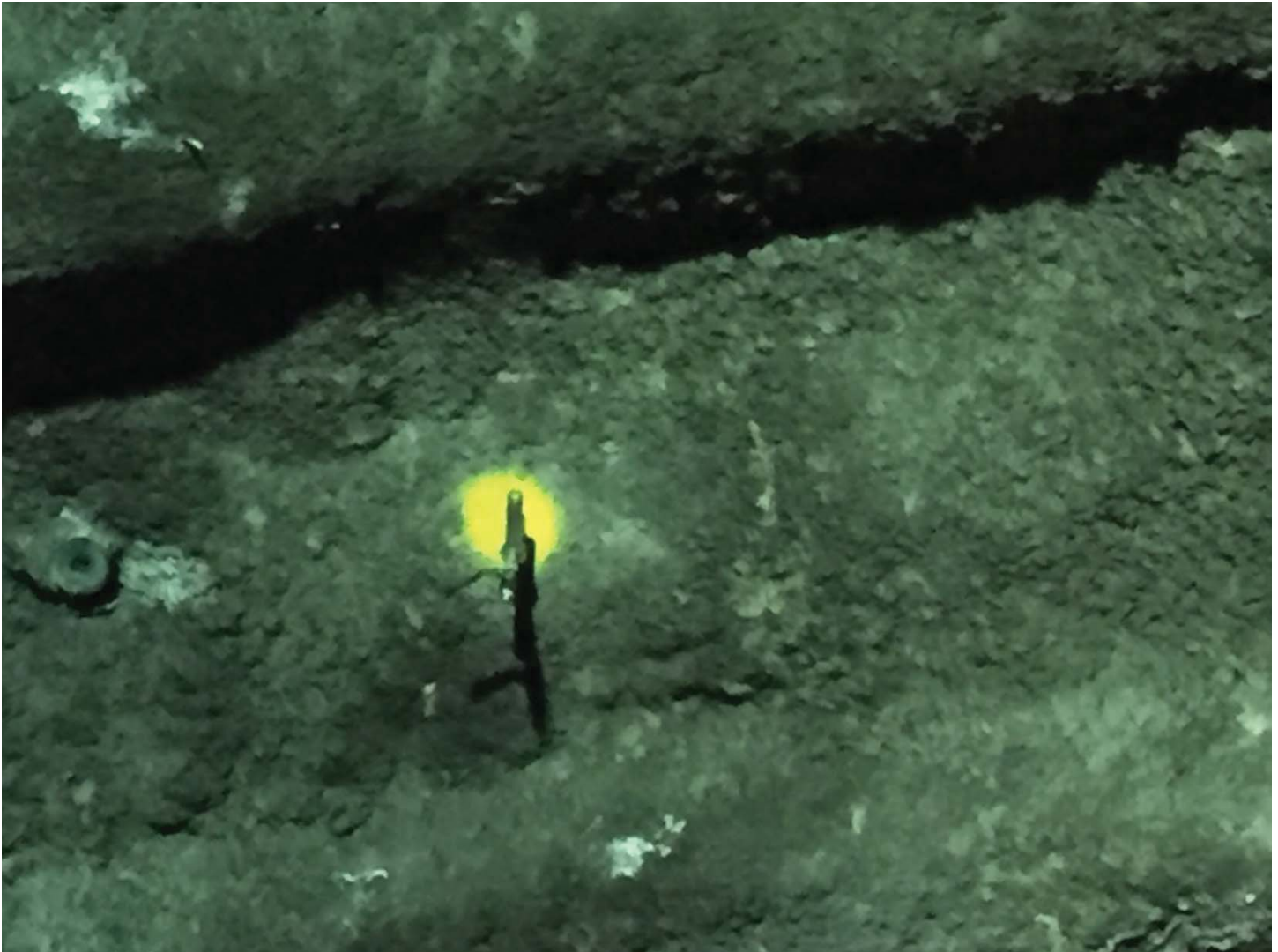
Figure 7: Hole after the solution is applied. After ample time to dry, the injection cylinder is removed, and the remaining hole filled. The cement finished is flush with the tunnel liner.
