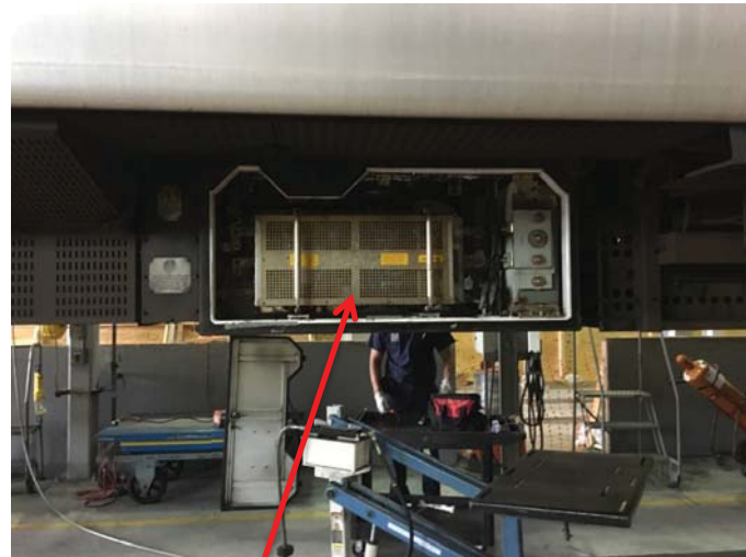
Exhibit 2: Traction Power Unit reinstalled.
