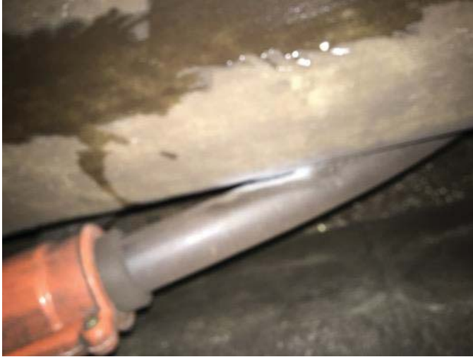
FIGURE 5 – A1 047+50 TO A1 050+50 - TROUGH/INVERT DRAIN CLOGGED
