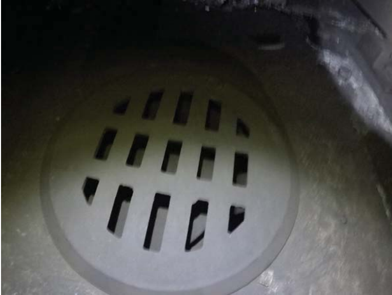
Figure 2: Drain obstructed by floating slab "puck" at G1 338+00.
