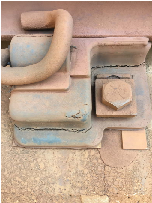
Figure 1: Defective elastic fastener
