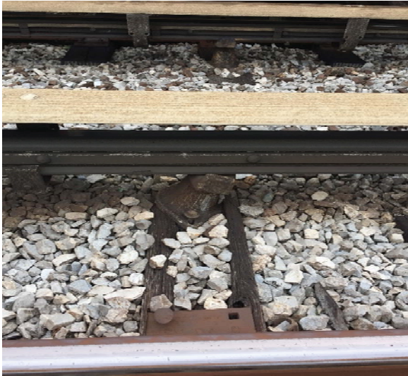
Figure 1: Non-holding third rail insulator support at E1 411+50.
