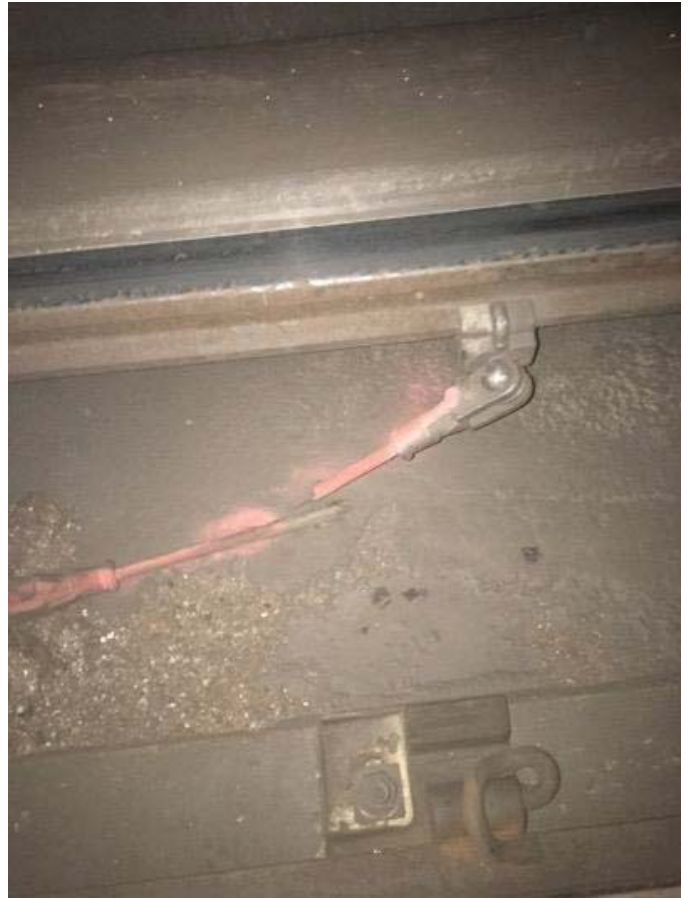
FIGURE 2 – A1 019+00 - 3 RD RAIL TIE ANCHOR BROKEN
