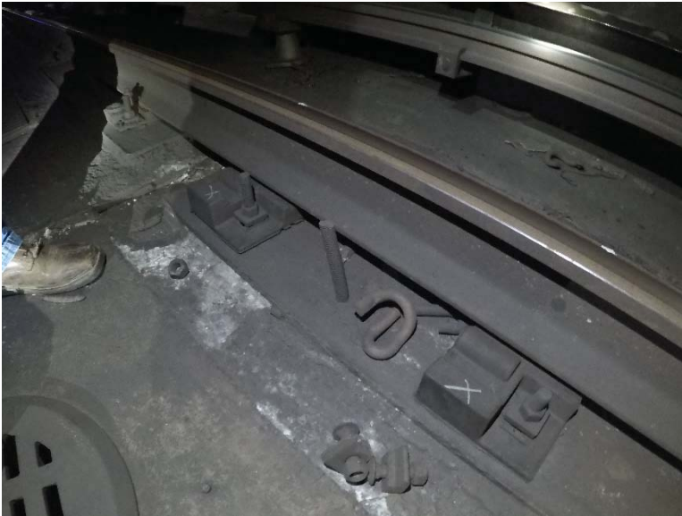
Figure 1: Defective Fasteners at G1 338+00.
