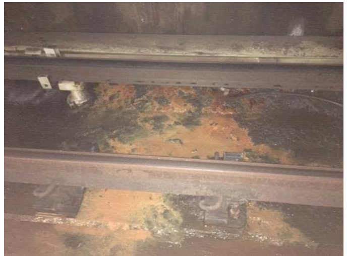
FIGURE 4 – A1 047+50 TO A1 048+00 - STANDING WATER AND CAKED MUD SURROUNDING 3 RD RAIL INSULATORS
