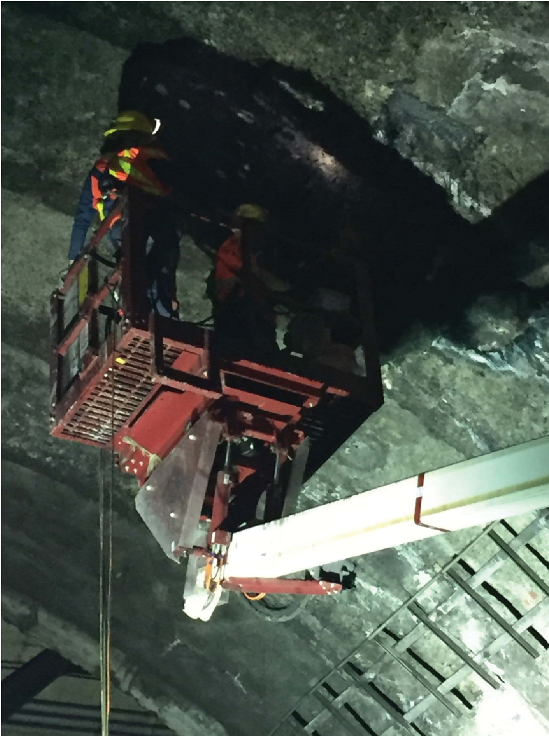
Figure 6: Crews in hi-rail bucket truck preparing to inject the solution into holes.
