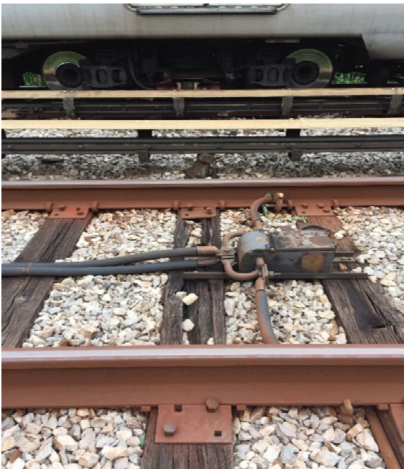
Figure 2: Defective non-supporting cross-tie allowing third rail insulator to collapse at E1 411+50.
