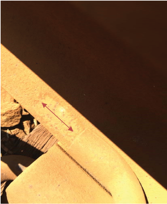
Figure 2: Pandrol mark on rail indicating lateral movement
