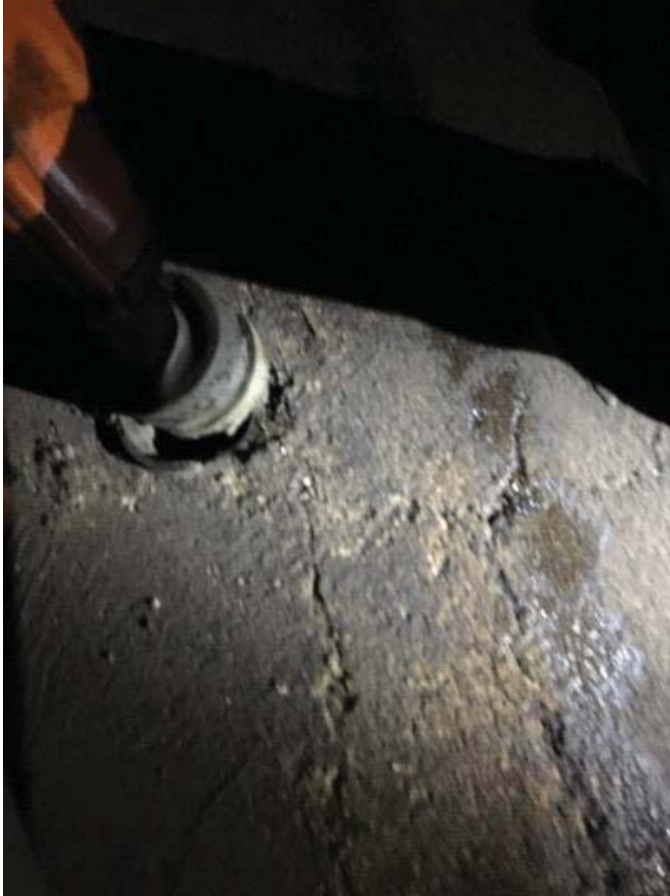
FIGURE 9 – A1 057+00 - CONDUIT STUB-UP BROKEN; NEEDS NEW OZ GEDNEY BUSHING
