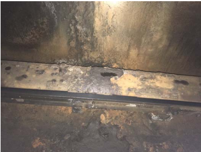
FIGURE 3 – F1 174+50 – WATER LEAKING FROM TUNNEL CEILING ONTO 3 RD RAIL COVER BOARD.
