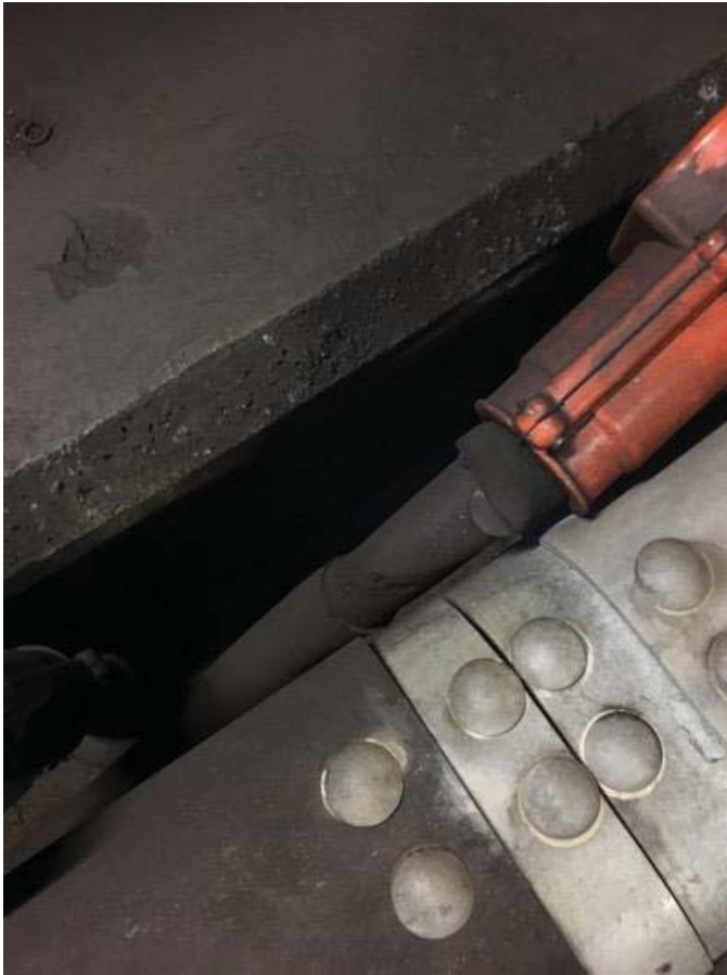
FIGURE 1 – A1 015+00 - CONDUIT STUB-UP BROKEN AND NEEDS NEW OZ GEDNEY BUSHING.
