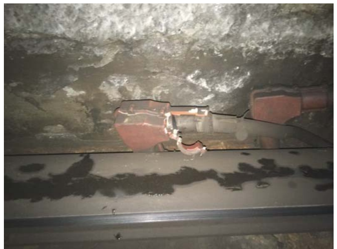
FIGURE 4 - C1 277+00 – ONE BROKEN ORANGE BOOT POWER CONNECTION ASSEMBLY
