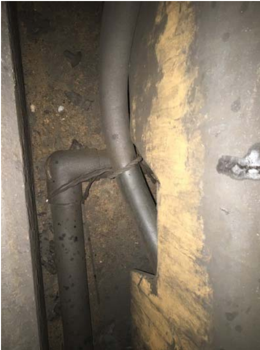
FIGURE 1 - C1 265+00 – TEMPORARY ROPE ON CABLE TO LIFT IT OFF THE GROUND NEEDS REMOVAL AND KINDORF SHOULD BE USED.
