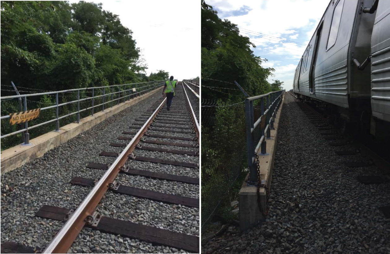
Figures 1 and 2: No clearance signage installed at J2 671+00 and a train passing this location
