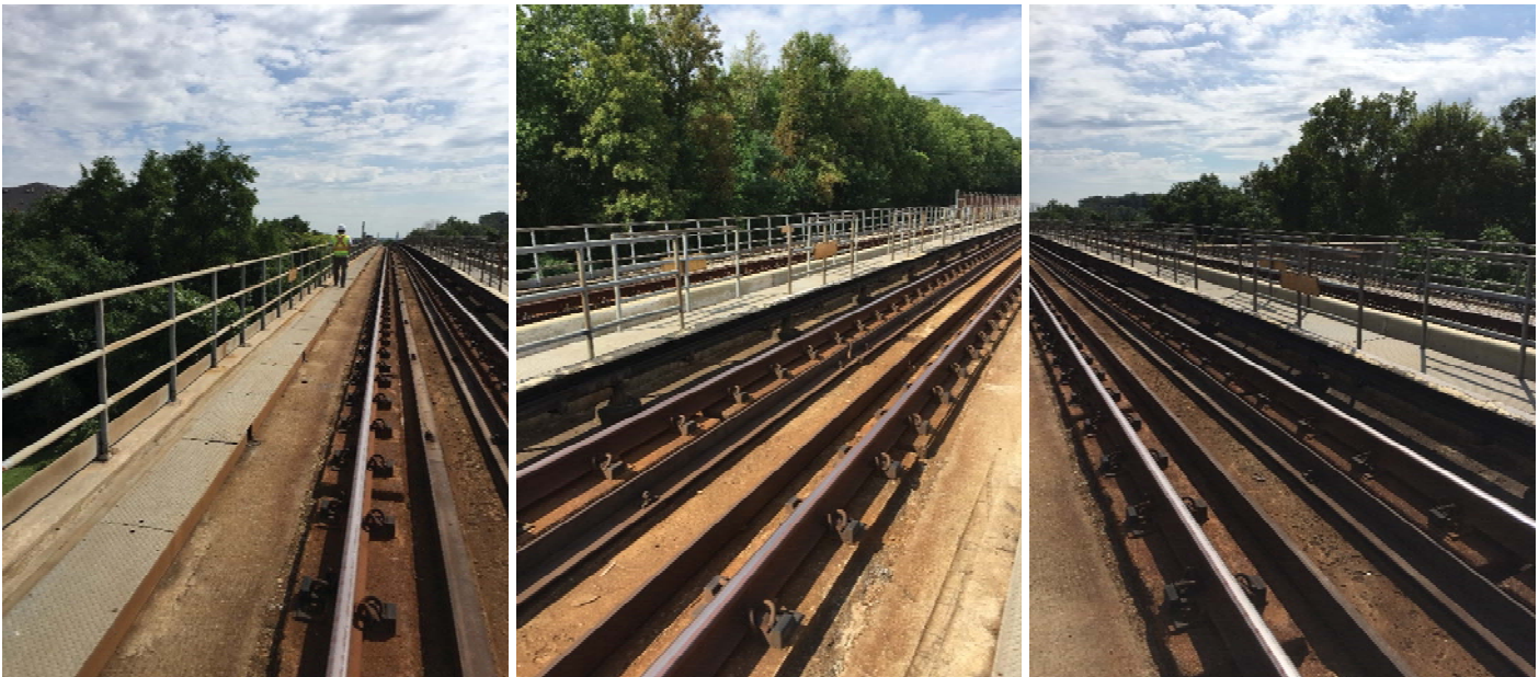
Figures 3, 4, and 5: Aerial structure at between CM 638+00 and 658+00 with no clearance signage installed on both sides
