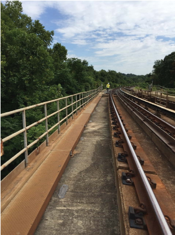
Figure 8: Aerial structure at between CM 622+00 and 628+00 with no clearance signage installed on both sides
