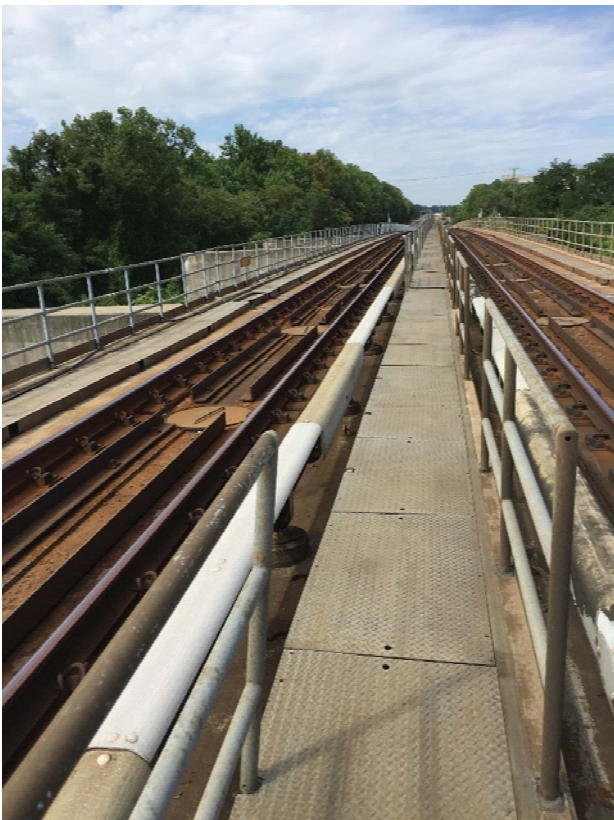
Figure 7: Missing handrail between CM 638+00 and 658+00.
