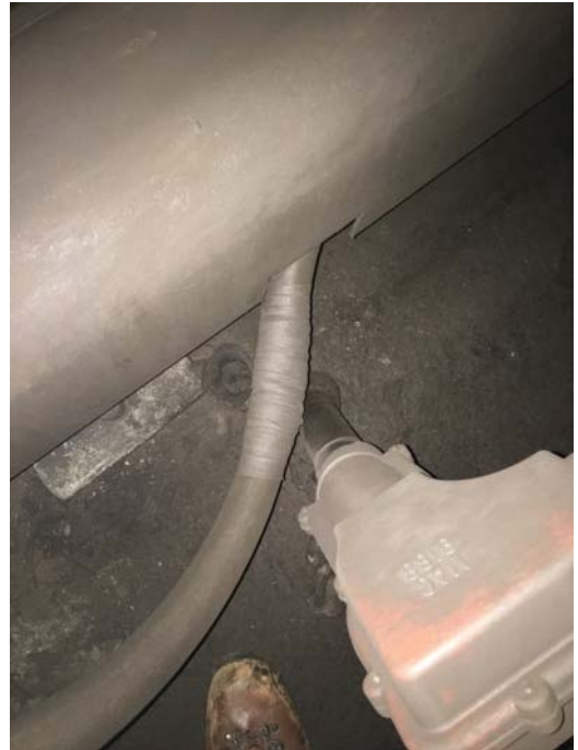
FIGURE 2 - C1 267+00 – FEEDER CABLE (PIGTAIL) HAS TEMPORARY REPAIR.
