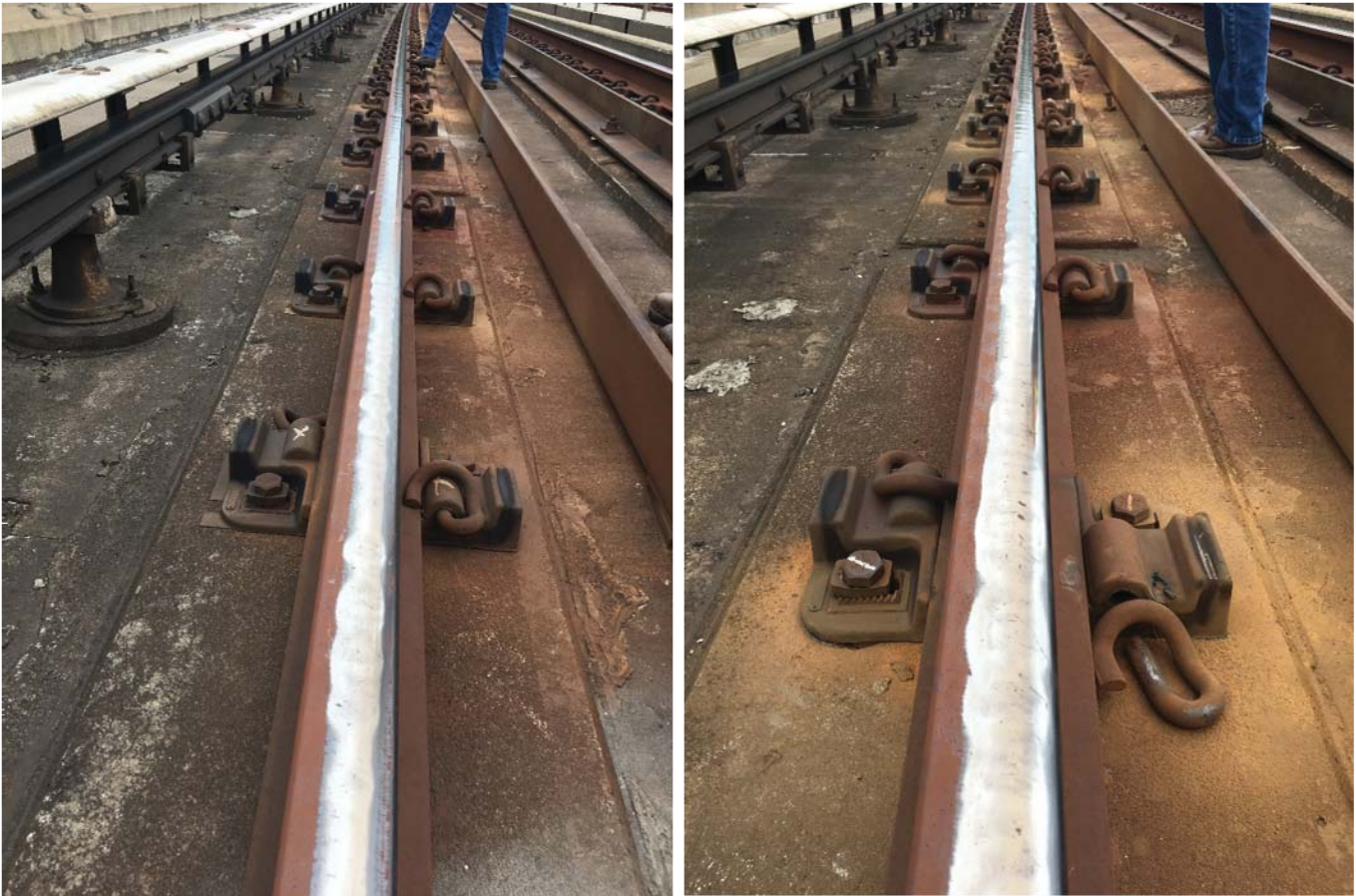
Figure 1: Rail Surface defects between F2 394+80 and 395+50.
