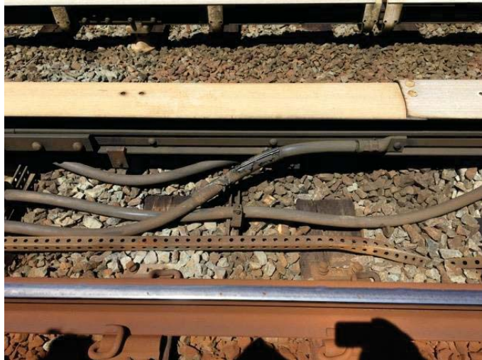
FIGURE 1 - J1 772+00 – EXPANSION CABLES ON GAUGE SIDE OF THIRD RAIL INSTALLED OFF THE GROUND WITH METAL KINDORF AND TEMPORARY REPAIR TO ONE EXPANSION CABLE.
