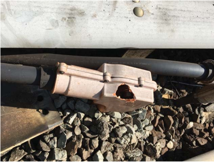
Figure 1: F2 398+00 – Broken Orange Boot Power Assembly
