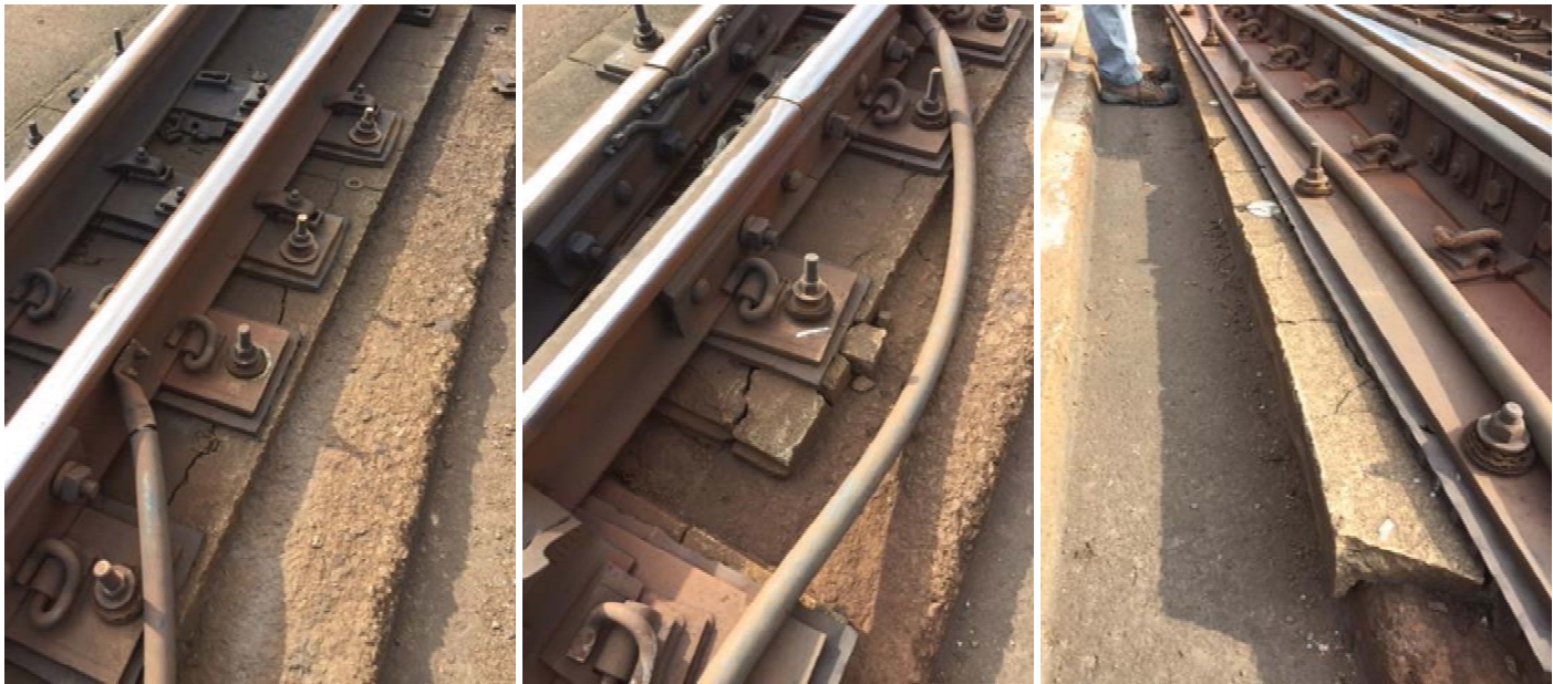
Figures 1, 2, and 3: 1B switch grout pad condition at C2 622+00
