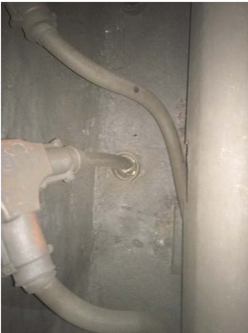
FIGURE 3 - C1 276+00 – FOUR CONDUIT STUB-UPS MISSING OZ GEDNEY BUSHINGS AND HEAT SHRINK
