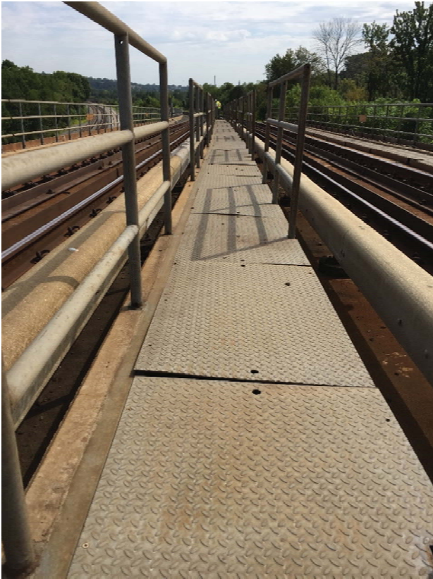
Figure 6: Loose and insecure walkway plates on the center catwalk between CM 638+00 and 658+00.
