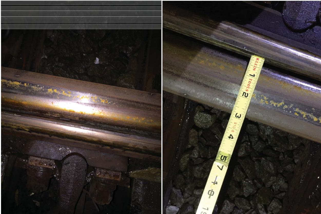
Figures 1 and 2: 5/8 inch gap between switch point and stock rail at the C98 1B switch on the outbound yard lead track adjacent to J2 538+50.
