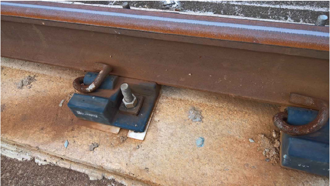
Figure 1: Fastener showing signs of degradation at D2 404+00
