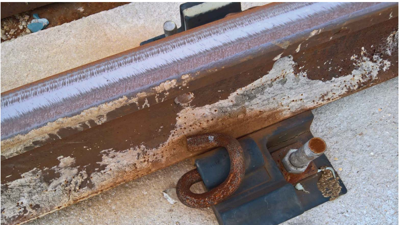
Figure 2: Fastener showing signs of degradation at D2 468+00
