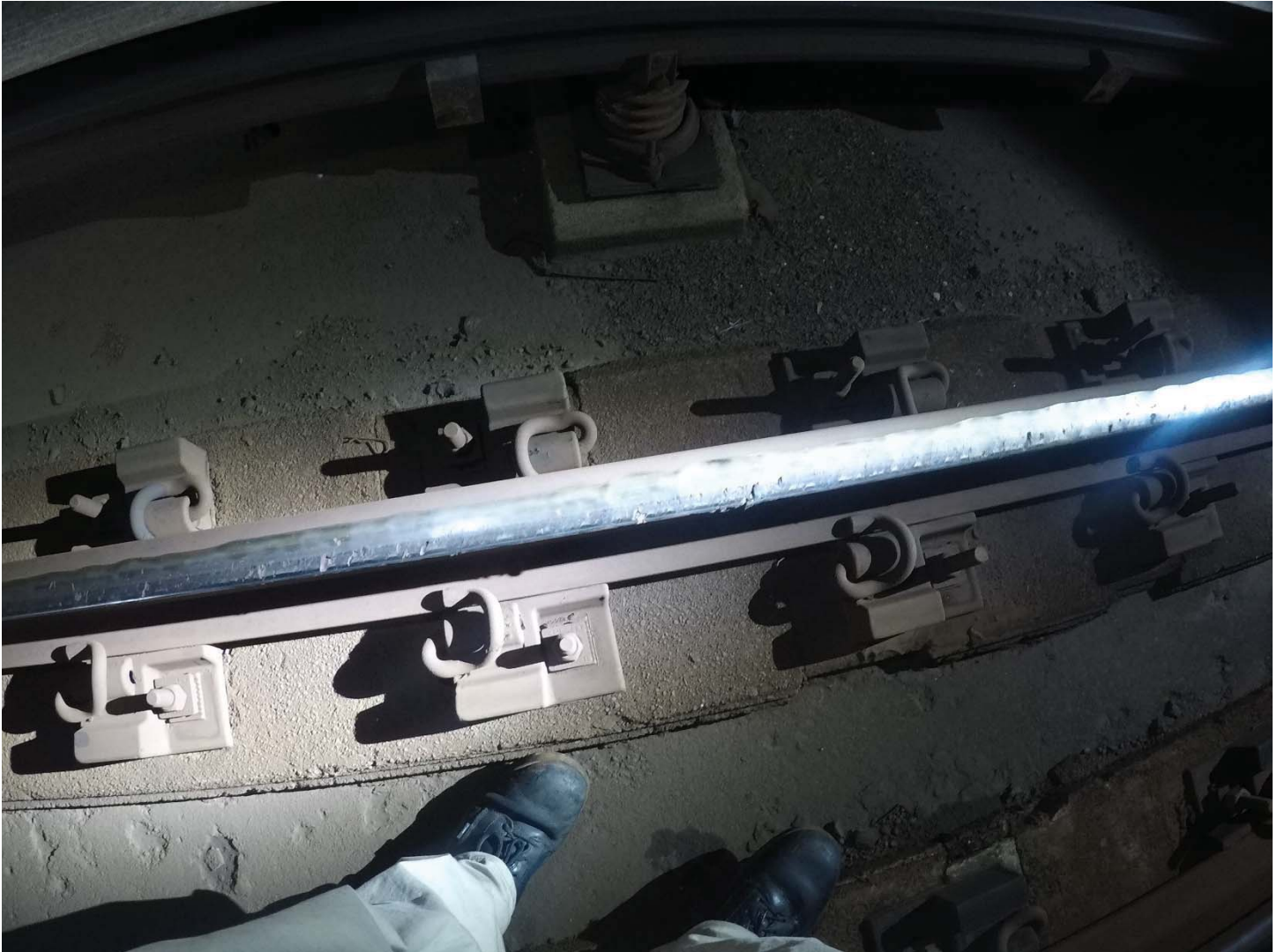
Figure 1: Spalling condition on the right rail at D1 283+50.
