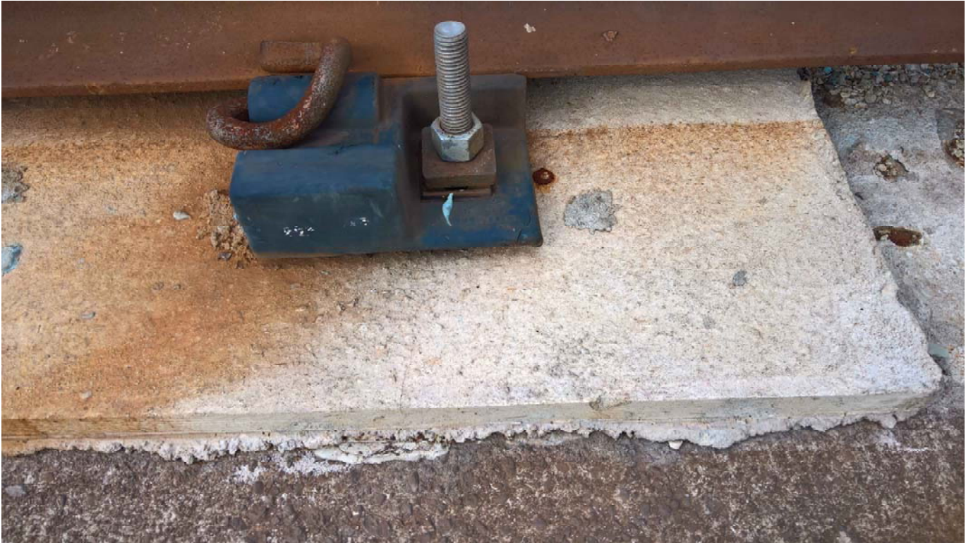
Figure 3: Fastener showing signs of degradation at D2 555+00
