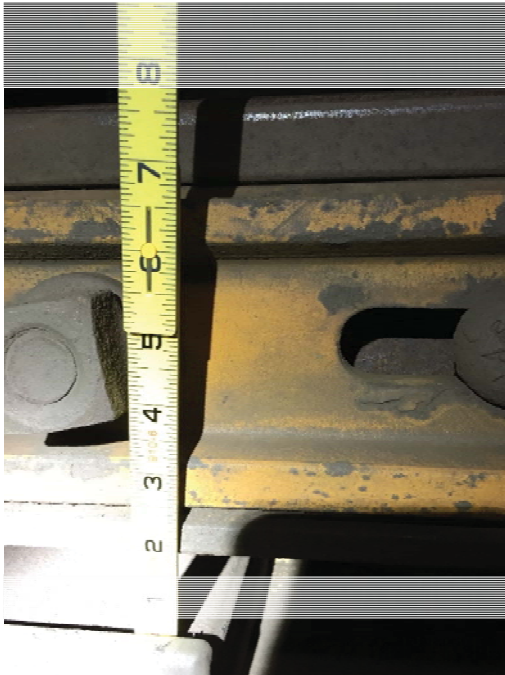
Figure 1: Rail joint at G1 409+30 suspended 1-7/8 inches from seat in elastic fasteners and not supported.
