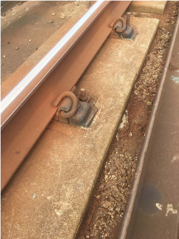
Figure 5: Deteriorating F-17 fasteners between B2 151+20 and 154+00.
