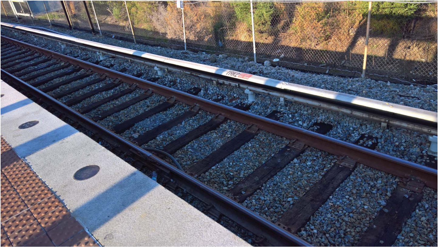
Figure 1: Ballast under third rail touching base of rail at New Carrollton Station (D13) at D2 598+50
