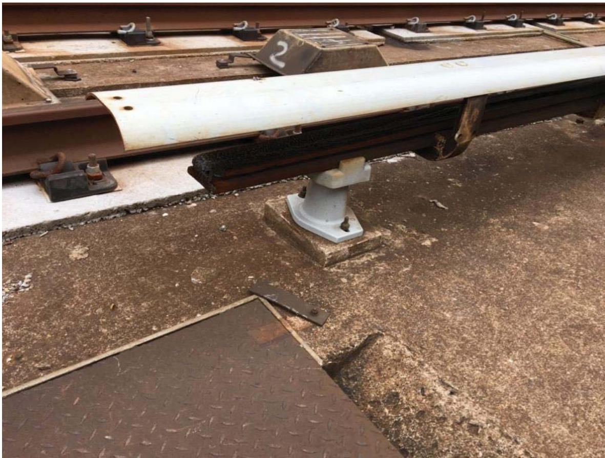
Figure 1: Third rail end approach arcing at C1 219+00.
