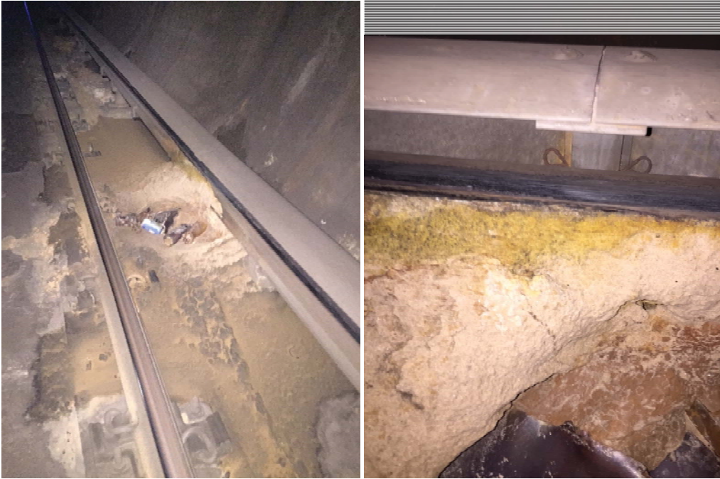
Figures 4 and 5: Mud/Silt contacting the third rail at G1 409+00, and showing signs of electric oxidation.
