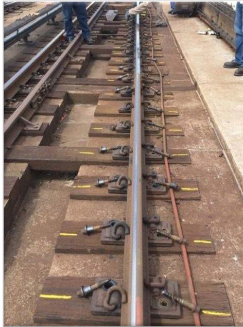
Figure 5-8 Loose spikes on track C1 between 40 th /46 th St stations
